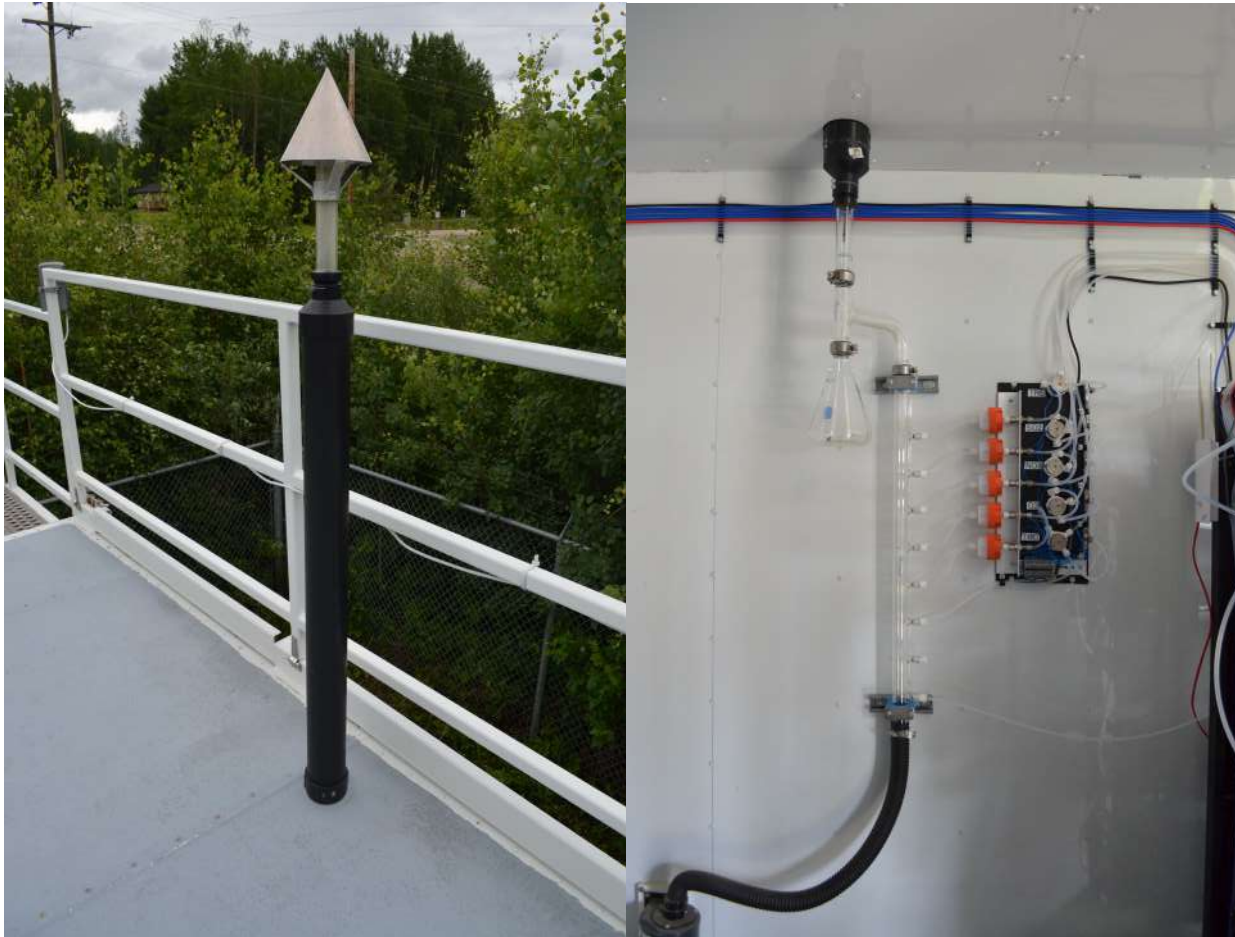
Figure 7.0 – Photo showing the inlet and sample manifold
