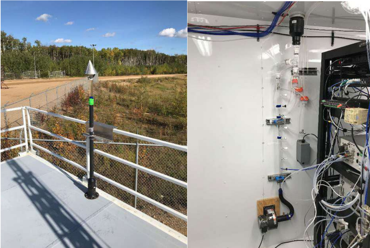
Figure 6.0 – Photo showing the inlet and sample manifold
