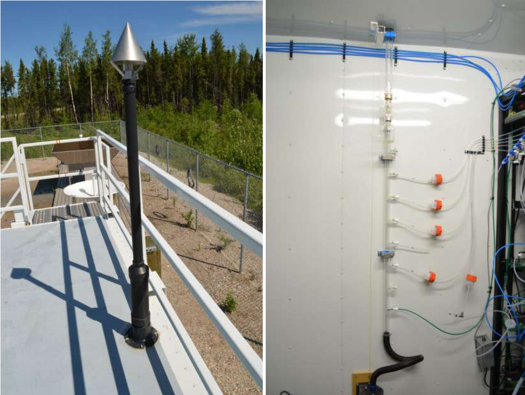
Figure 7.0 – Photo showing the inlet and sample manifold
