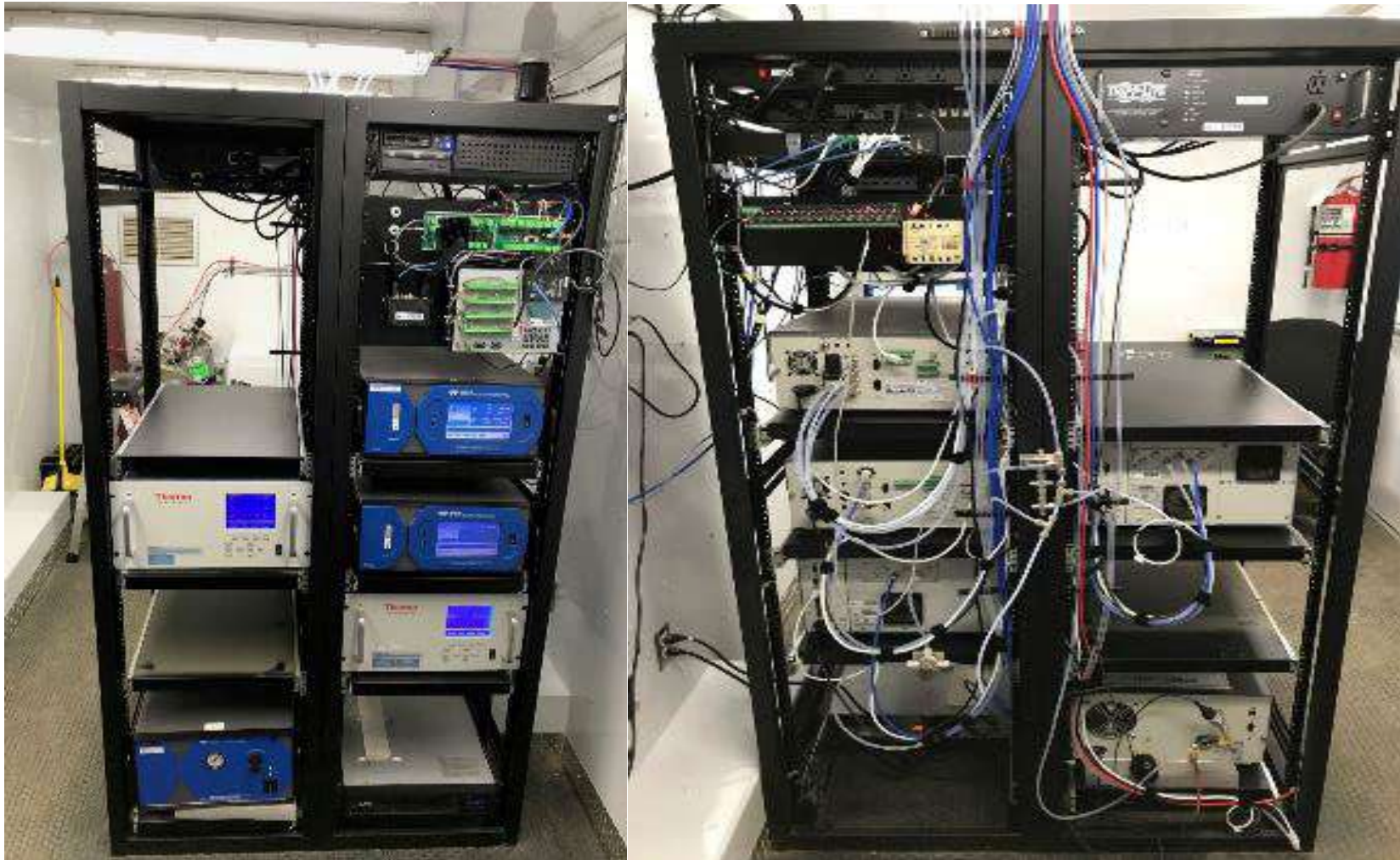
Figure 12 –Photo of the front and the back of instrument rack
