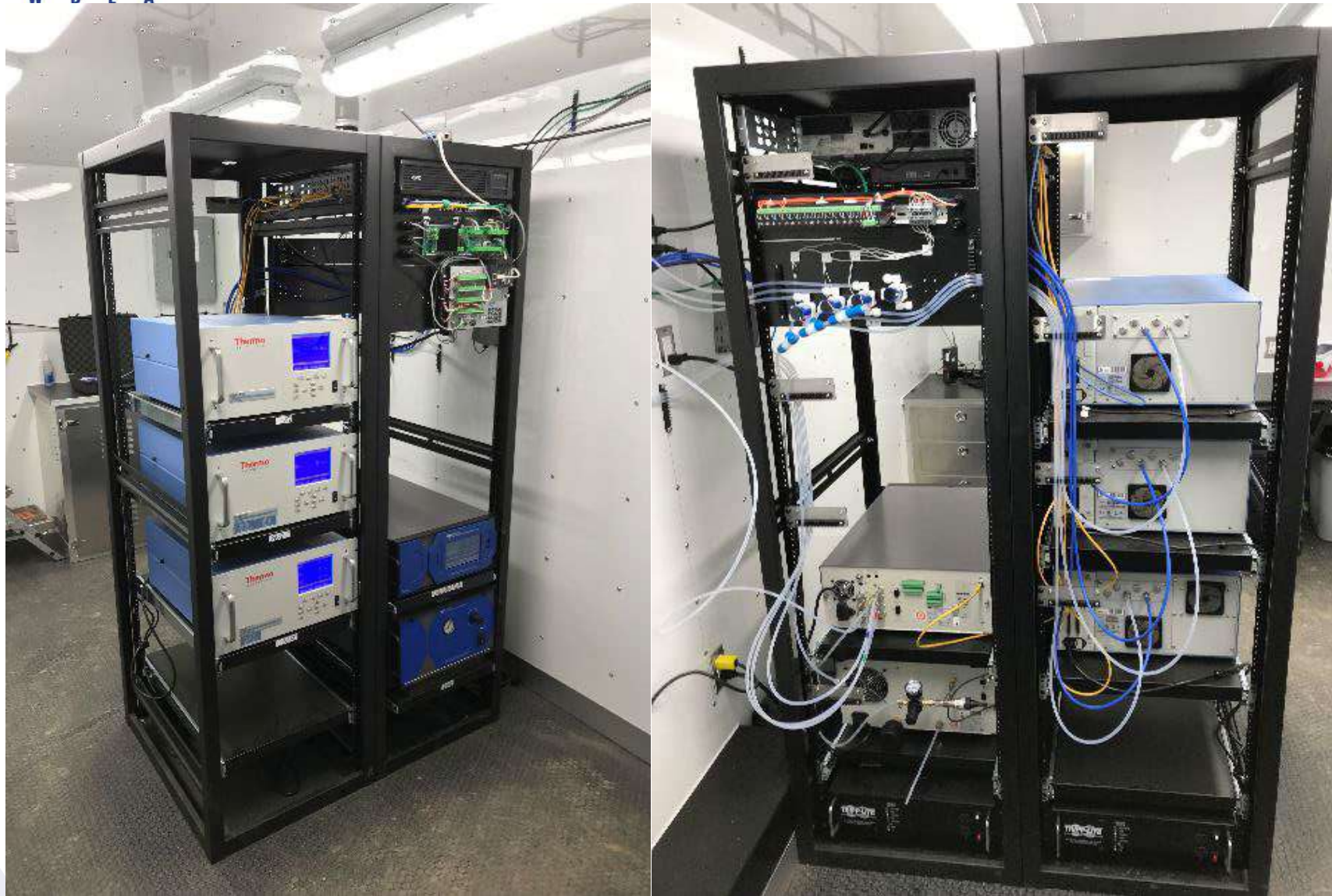
Figure 7.2 –Photo of front and back of instrument rack.
