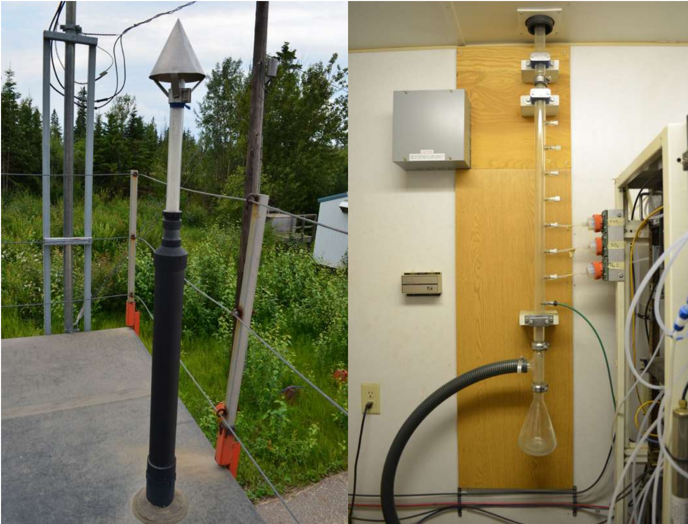
Figure 7.0 – Photo showing the inlet and sample manifold
