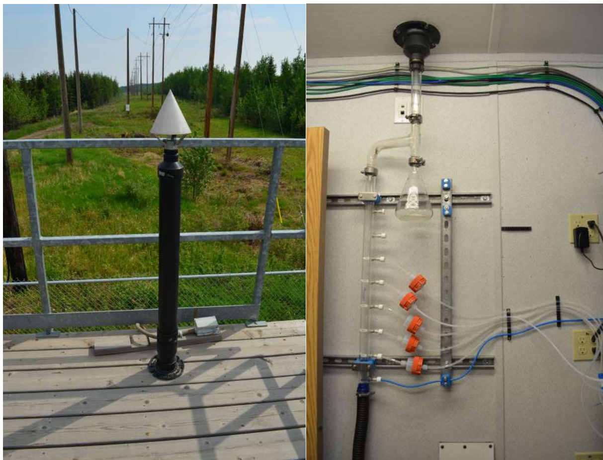
Figure 7.0 – Photo showing the inlet and sample manifold
