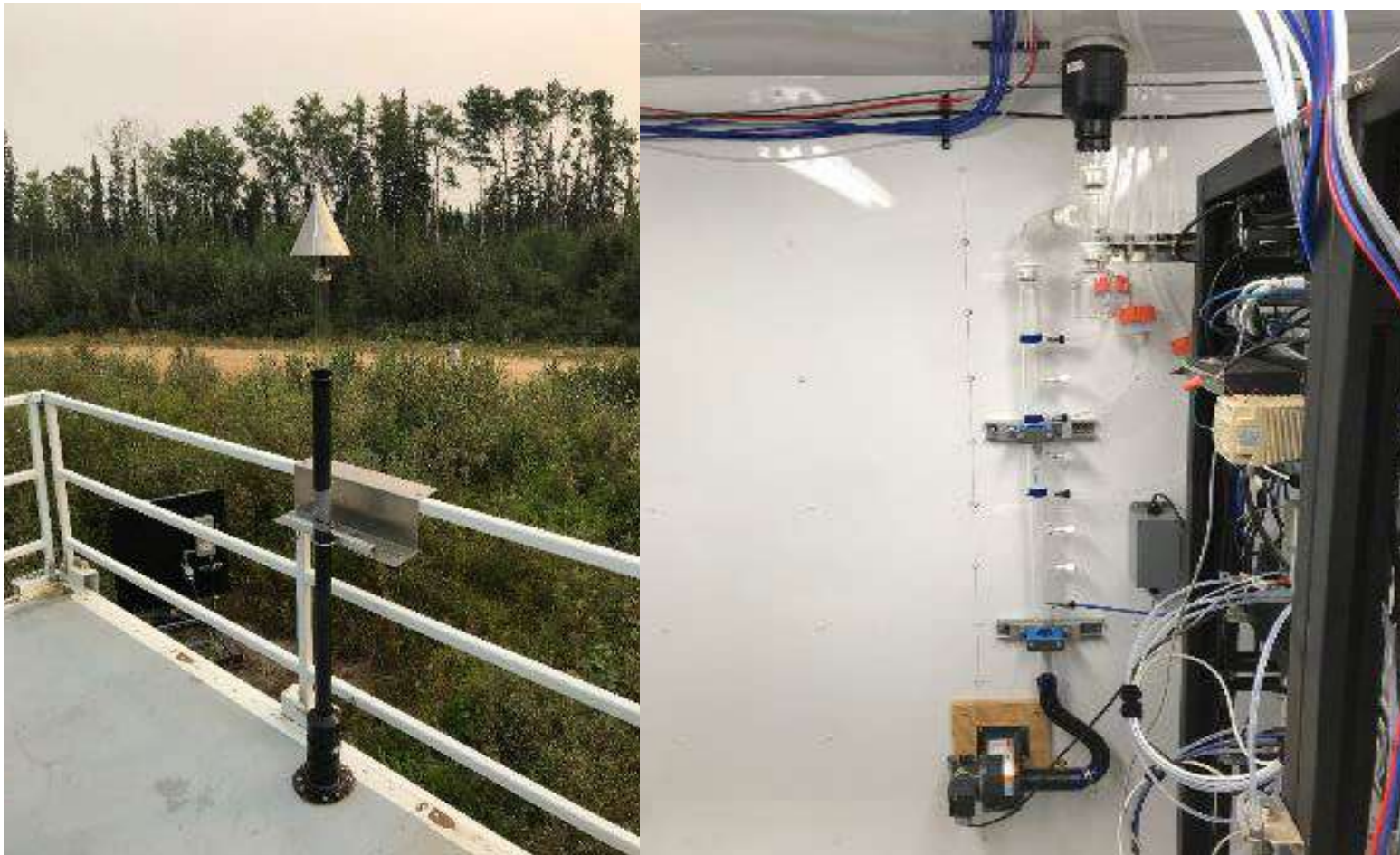
Figure 10 – Photo showing the inlet and sample manifold
