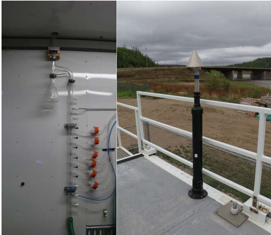
Figure 7.0 – Photo showing the inlet and sample manifold
