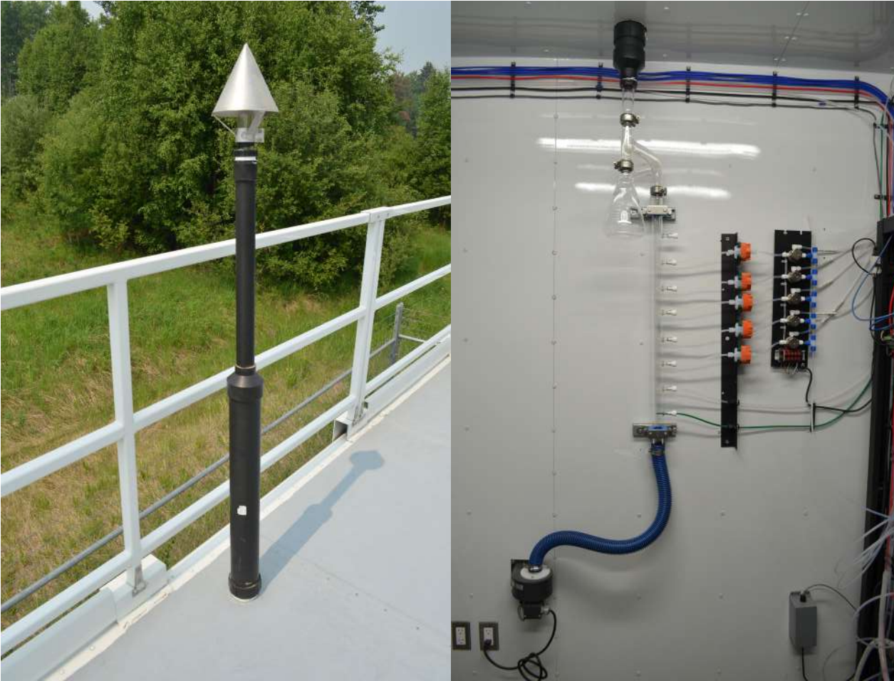
Figure 7.0 – Photo showing the inlet and sample manifold.
