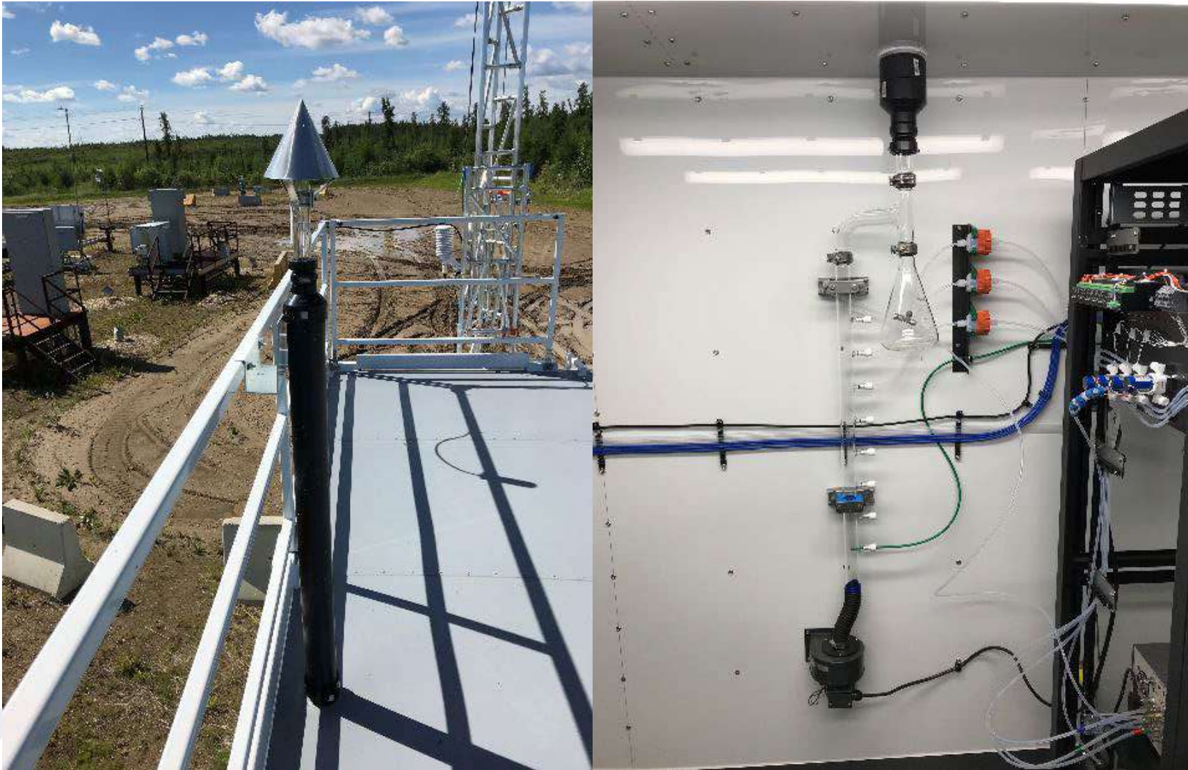
Figure 7.0 – Photo showing the inlet and sample manifold.
