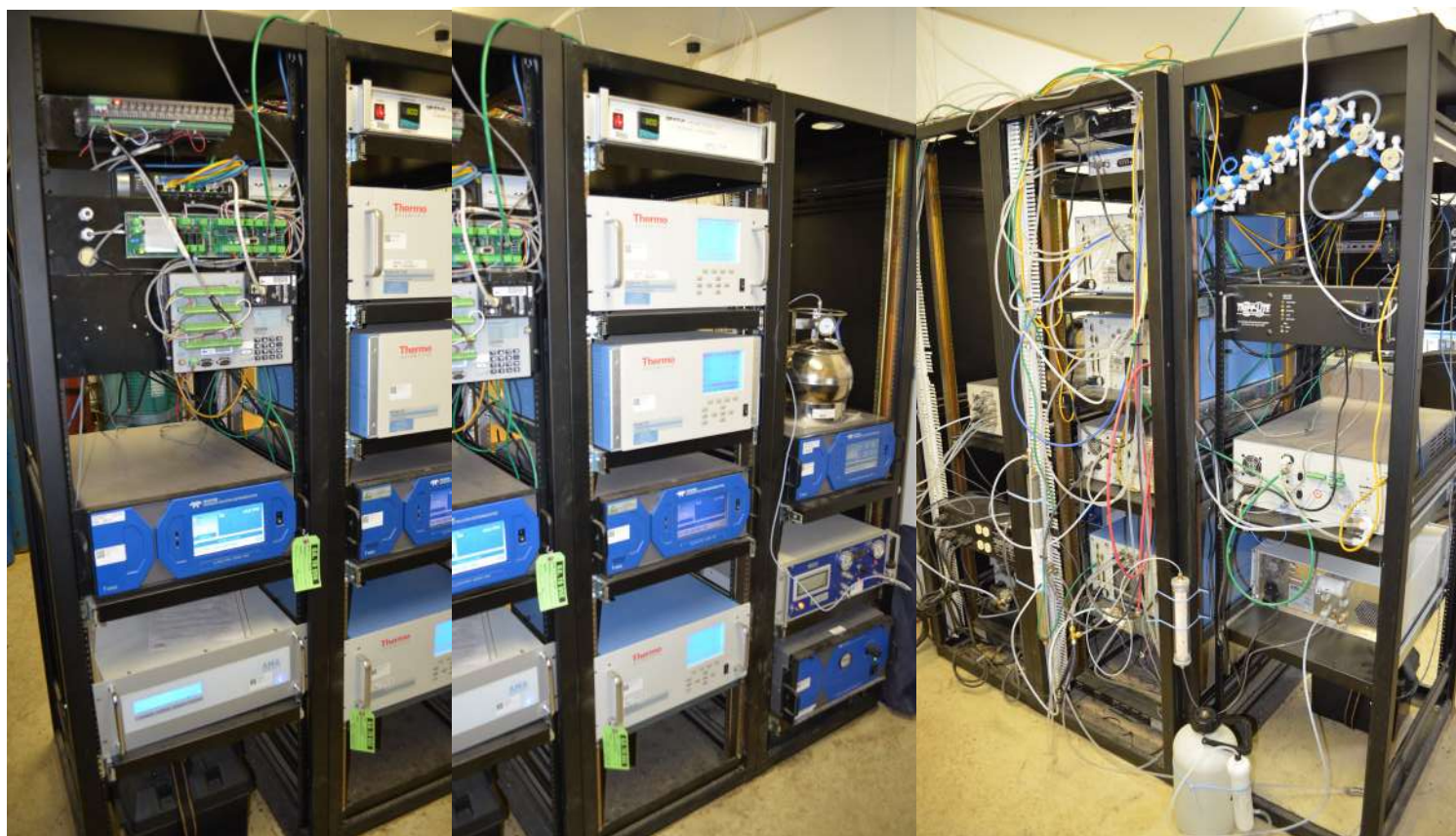
Figure 7.2 –Photo of the front and the back of instrument rack
