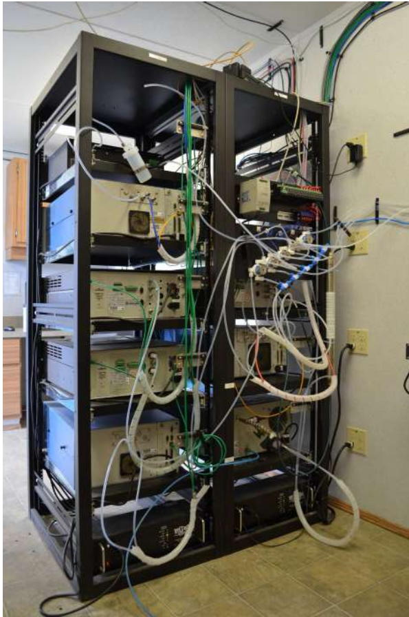
Figure 7.2 –Photo of the front and the back of instrument rack
