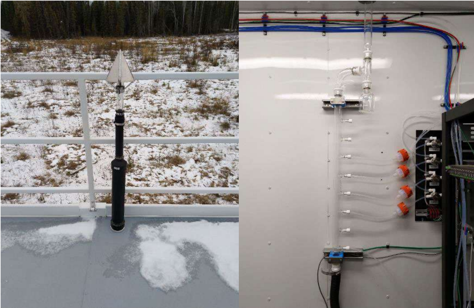
Figure 7.0 – Photo showing the inlet and sample manifold
