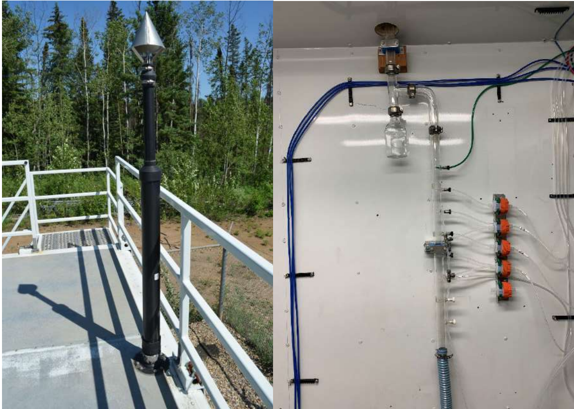
Figure 7.0 – Photo showing the inlet and sample manifold
