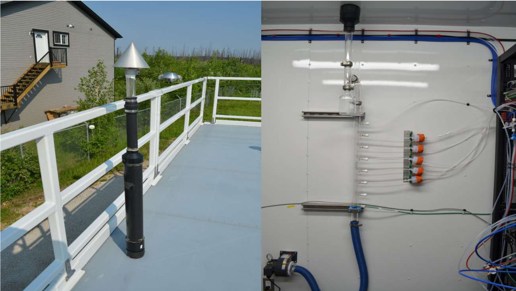
Figure 7.0 – Photo showing the inlet and sample manifold.
