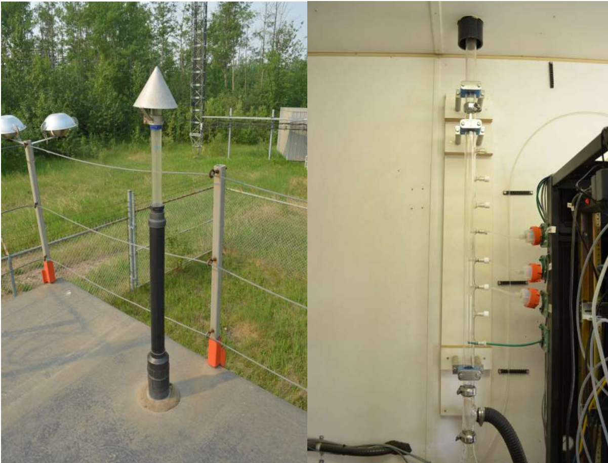
Figure 7.0 – Photo showing the inlet and sample manifold
