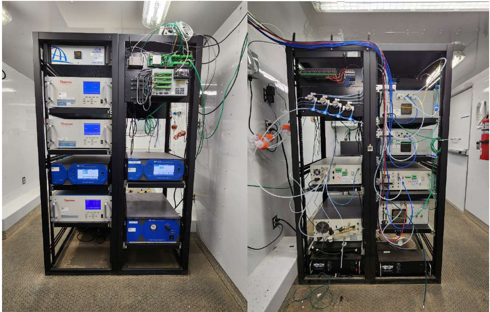
Figure 7.2 –Photo of the front and the back of instrument rack
