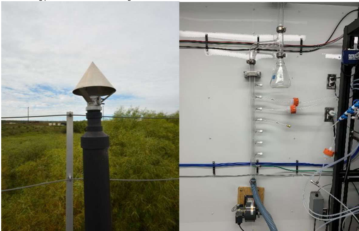
Figure 7.0 – Photo showing the inlet and sample manifold.
