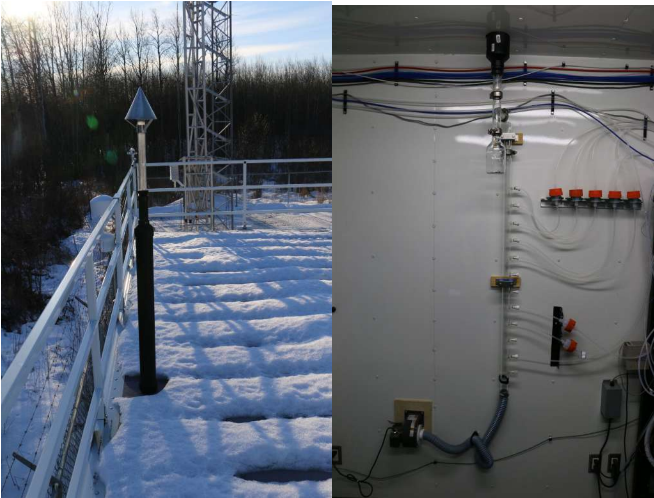
Figure 7.0 – Photo showing the inlet and sample manifold
