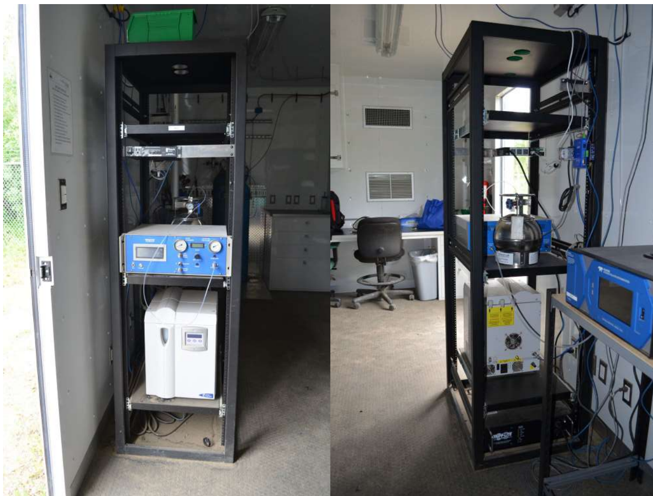
Figure 7.2 –Photo of the front and the back of instrument rack
