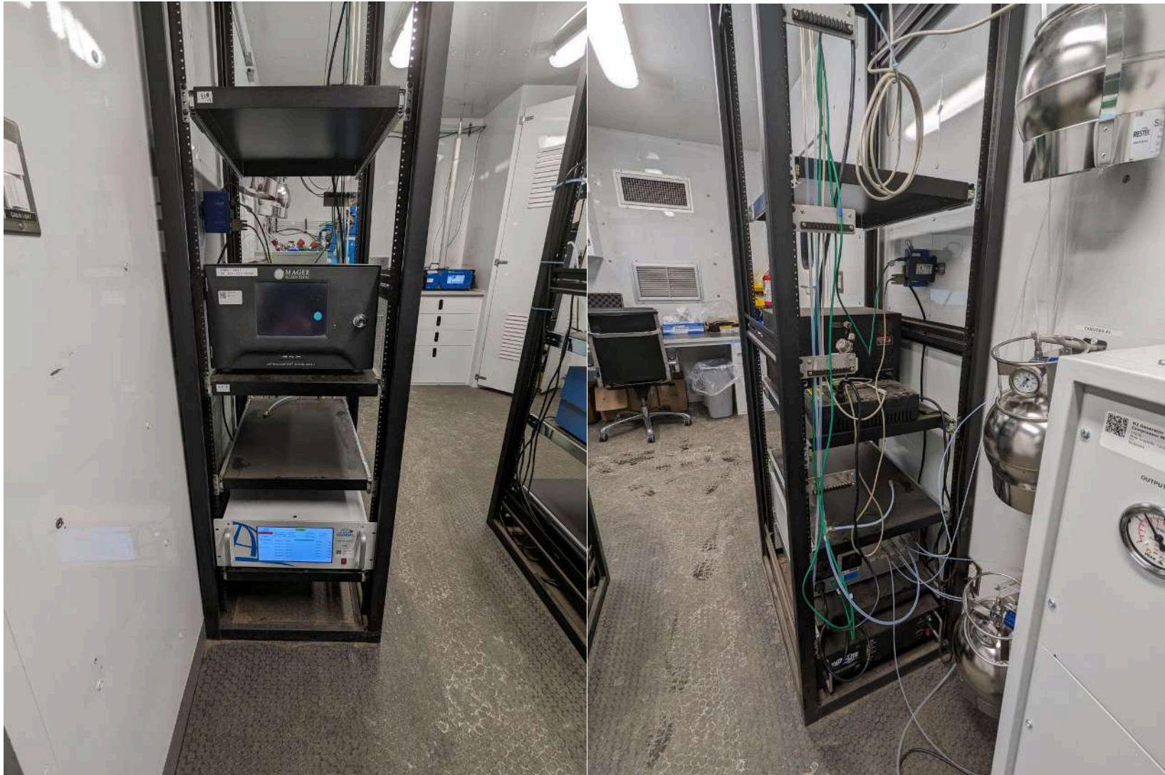
Figure 7.2 –Photo of the front and the back of the instrument rack
