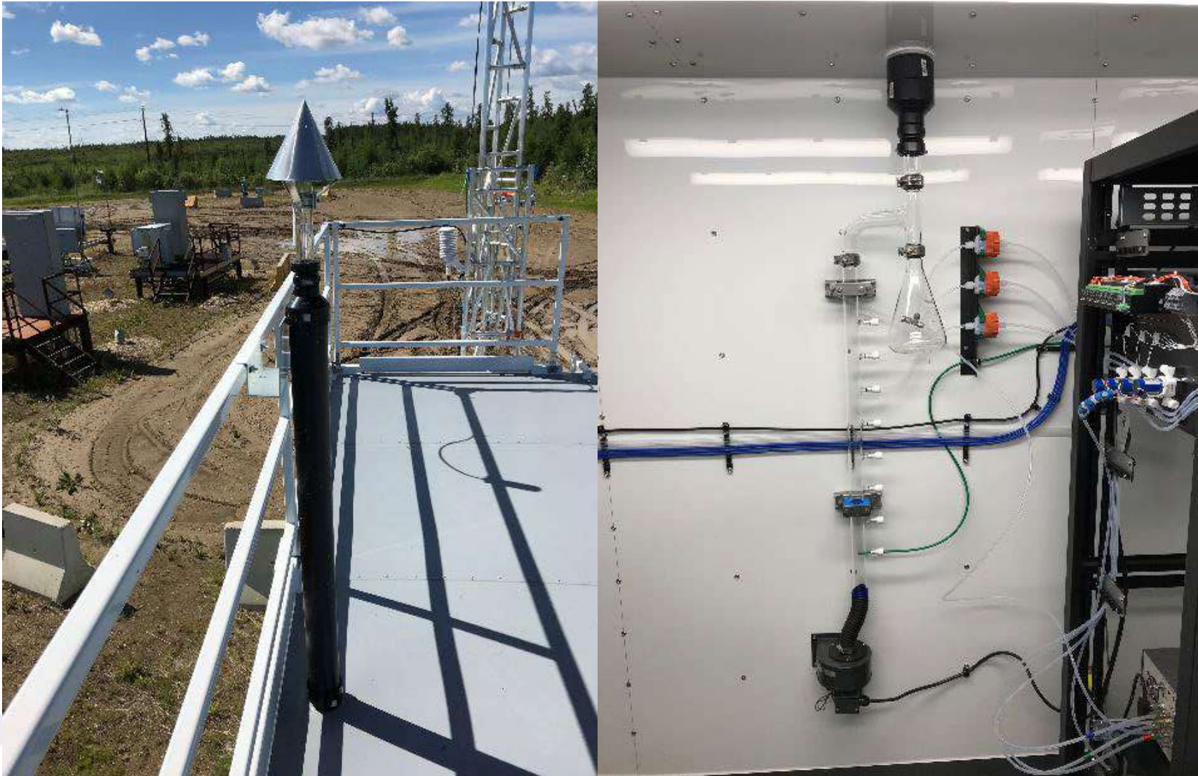
Figure 7.0 – Photo showing the inlet and sample manifold.
