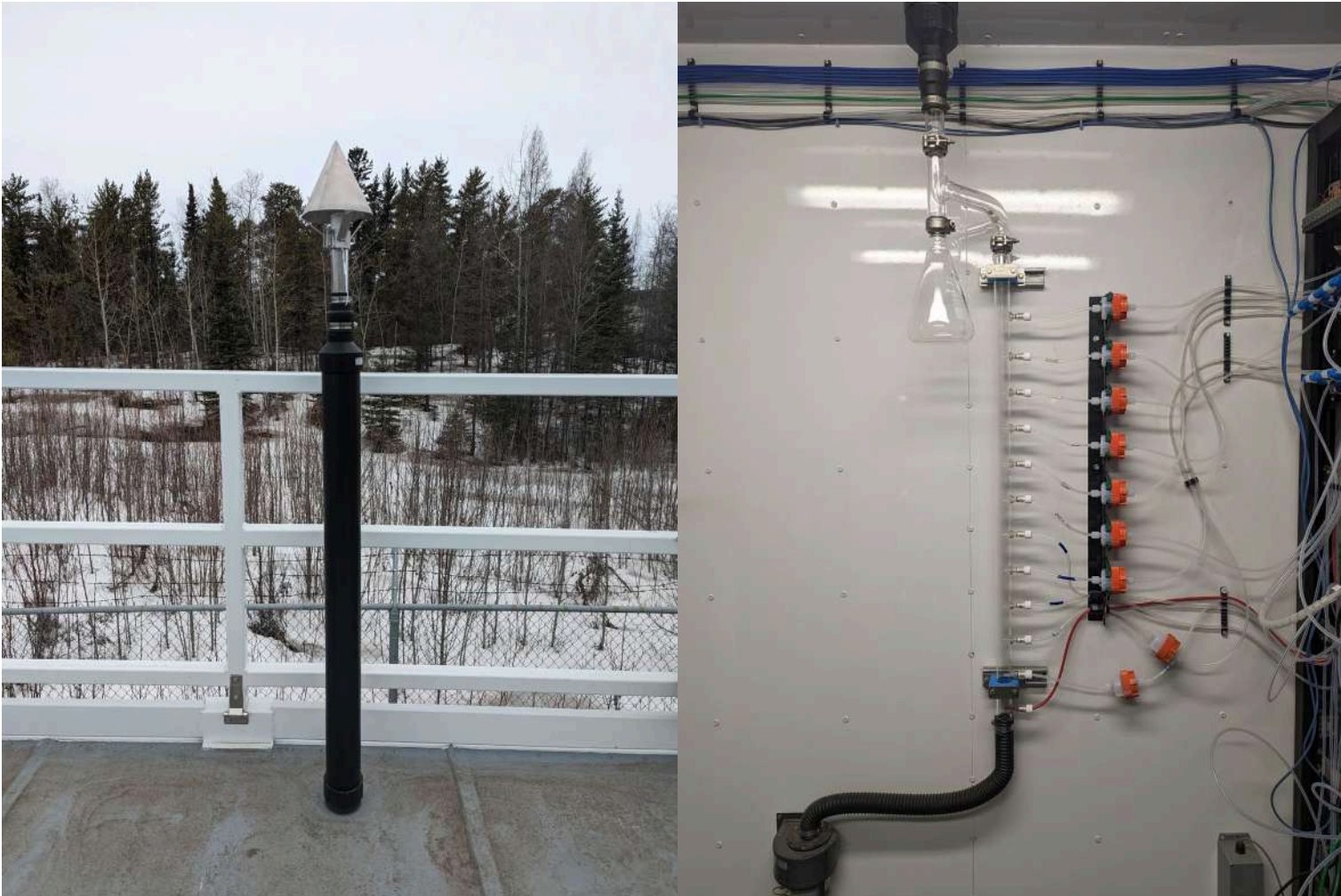
Figure 7.0 – Photo showing the inlet and sample manifold
