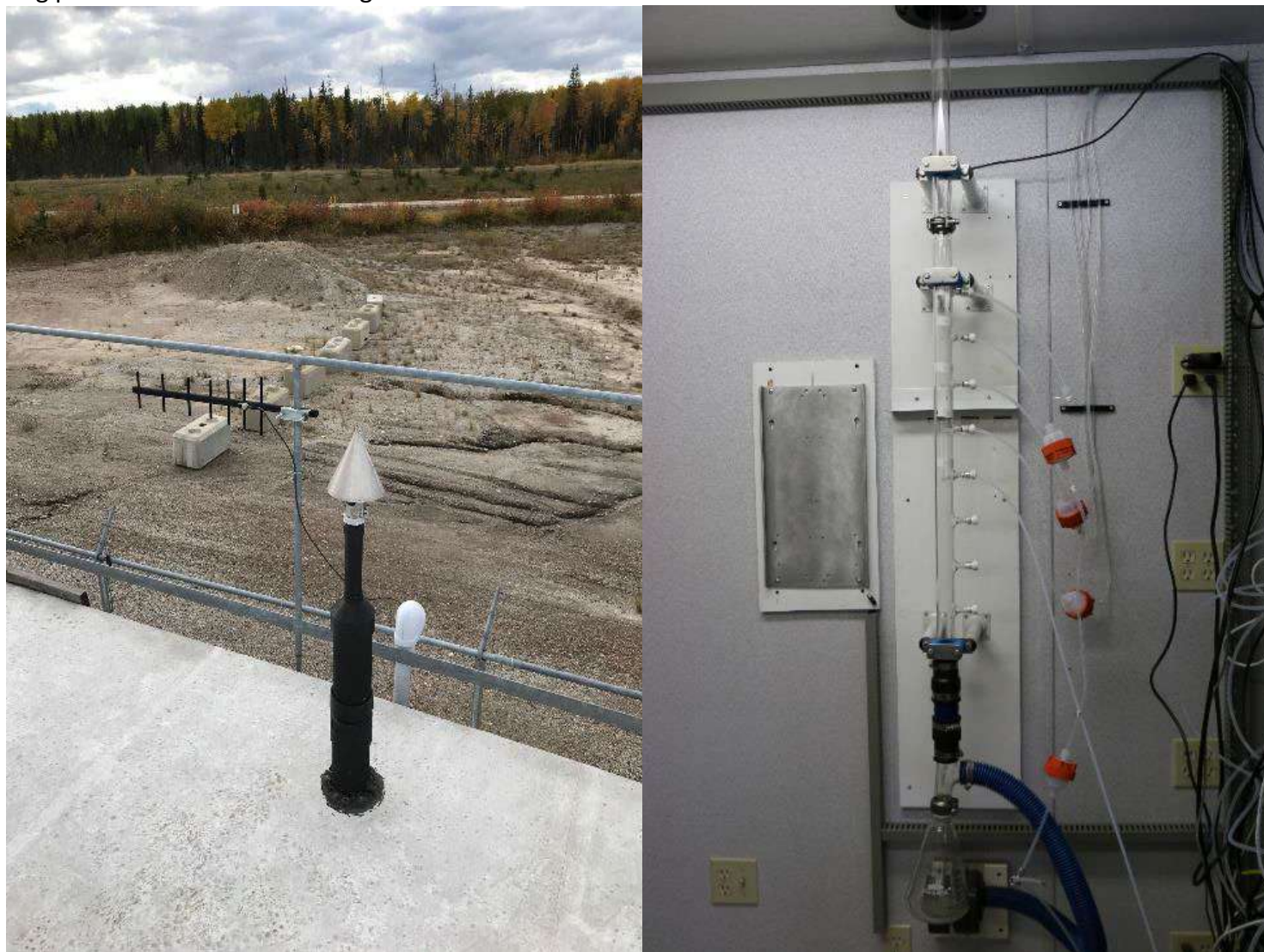
Figure 7.0 – Photo showing the inlet and sample manifold
