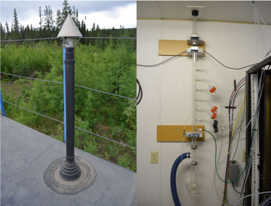
Figure 7.0 – Photo showing the inlet and sample manifold.
