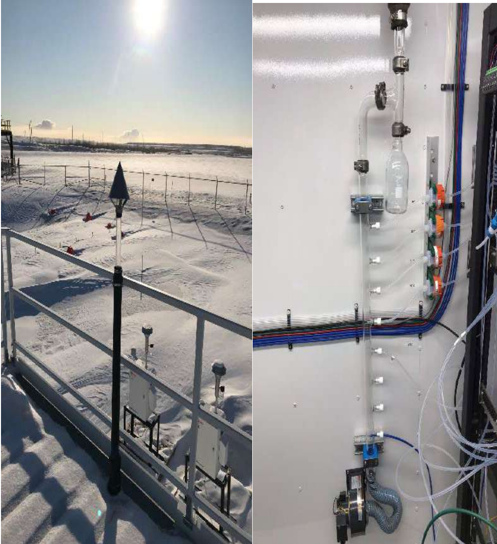
Figure 6.0 – Photo showing the inlet and sample manifold
