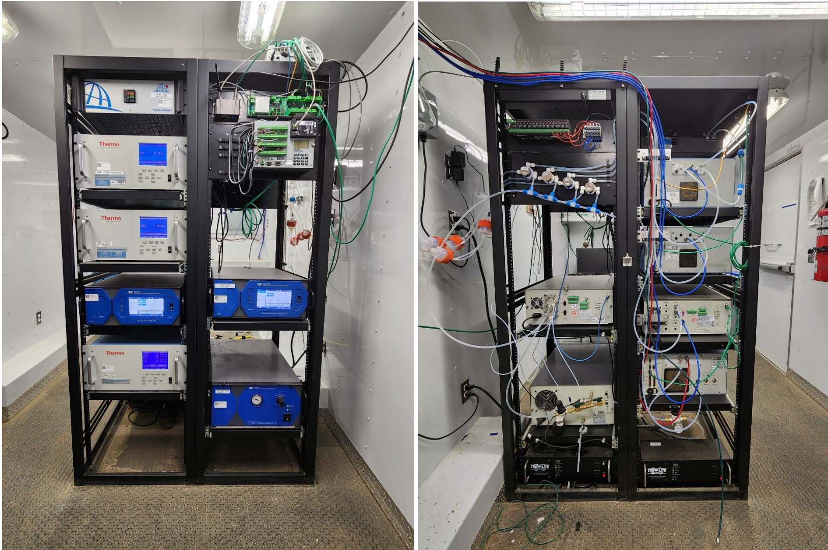
Figure 11 –Photo of the front and the back of instrument rack
