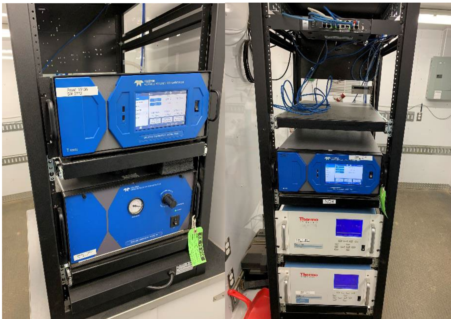
Figure 11 –Photo of the front and the back of instrument rack
