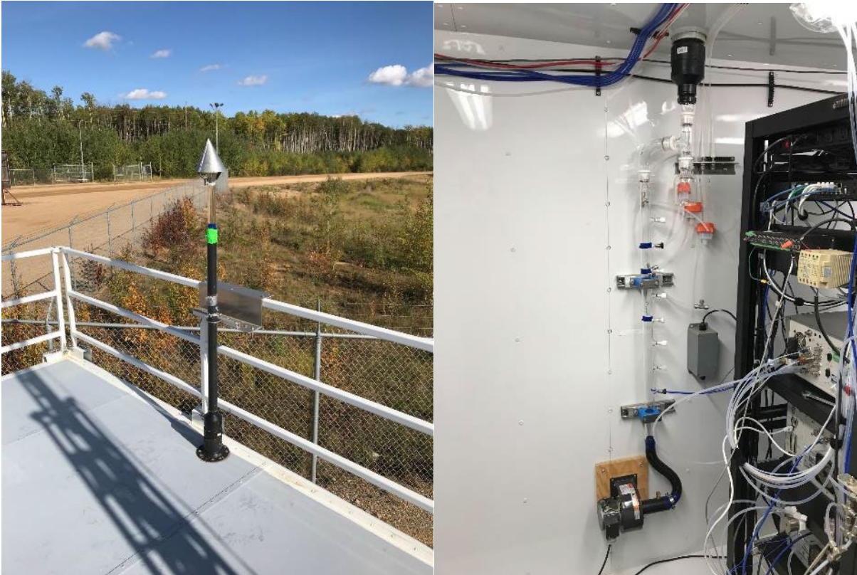
Figure 9 – Photo showing the inlet and sample manifold
