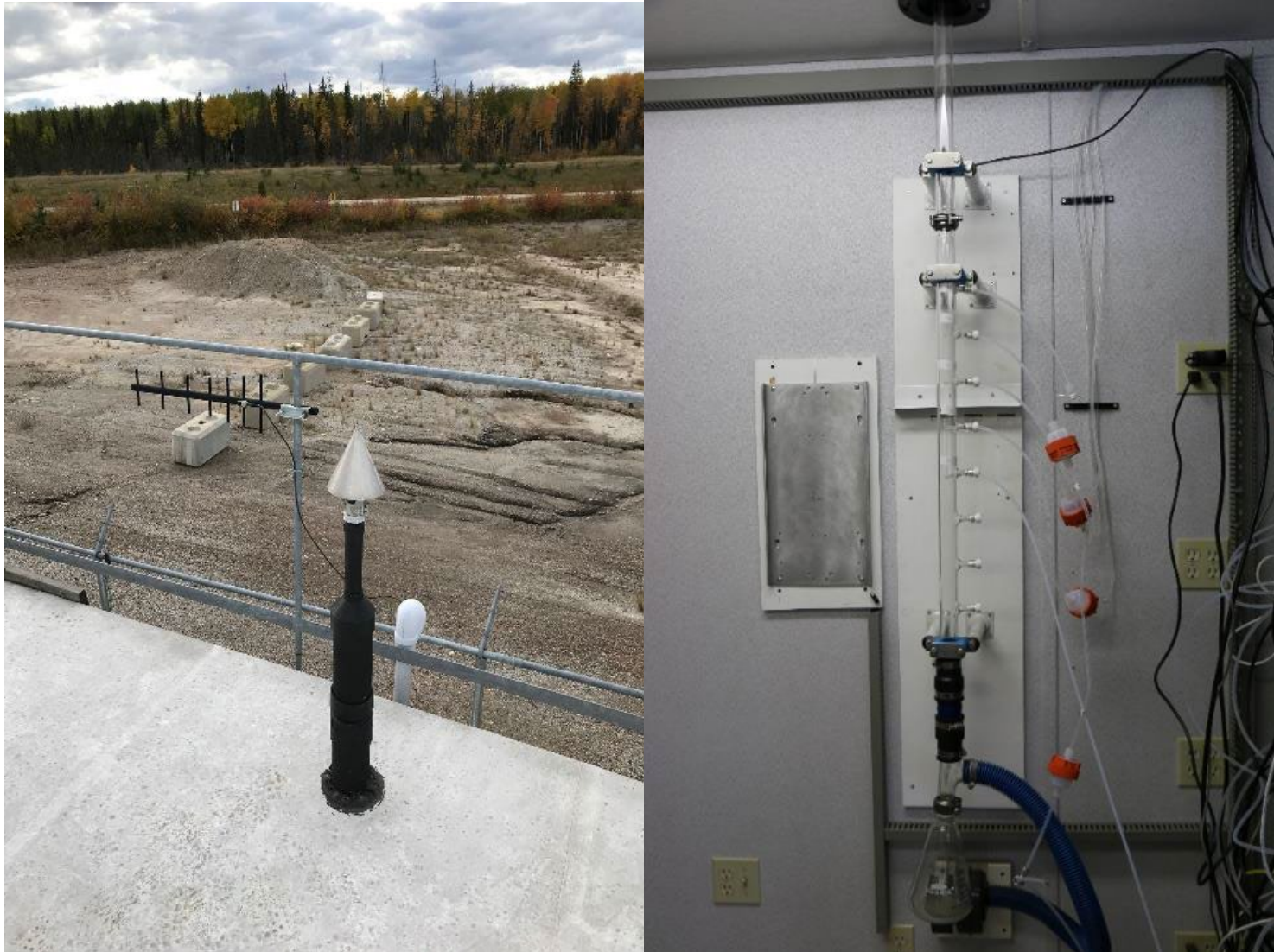
Figure 10 – Photo showing the inlet and sample manifold
