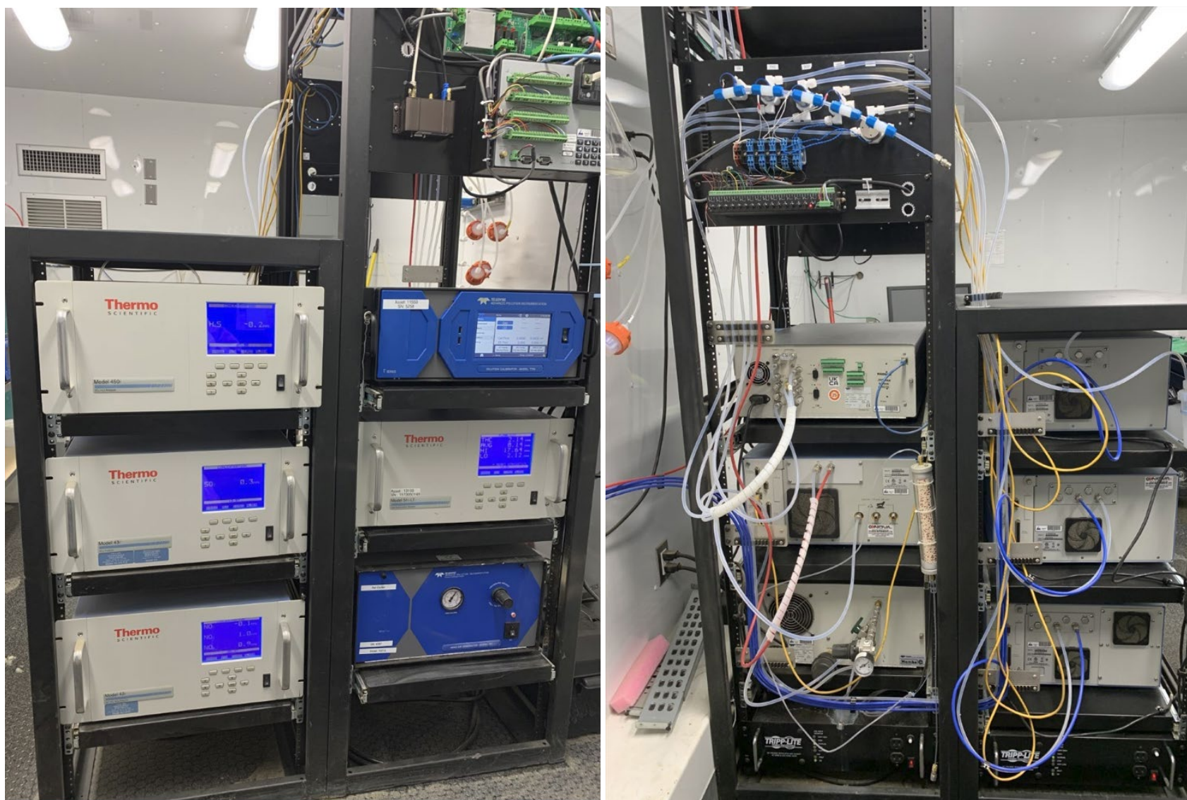
Figure 12 –Photo of the front and the back of instrument rack
