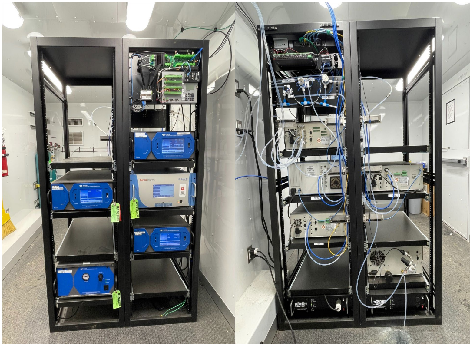
Figure 11 –Photo of the front and the back of instrument rack
