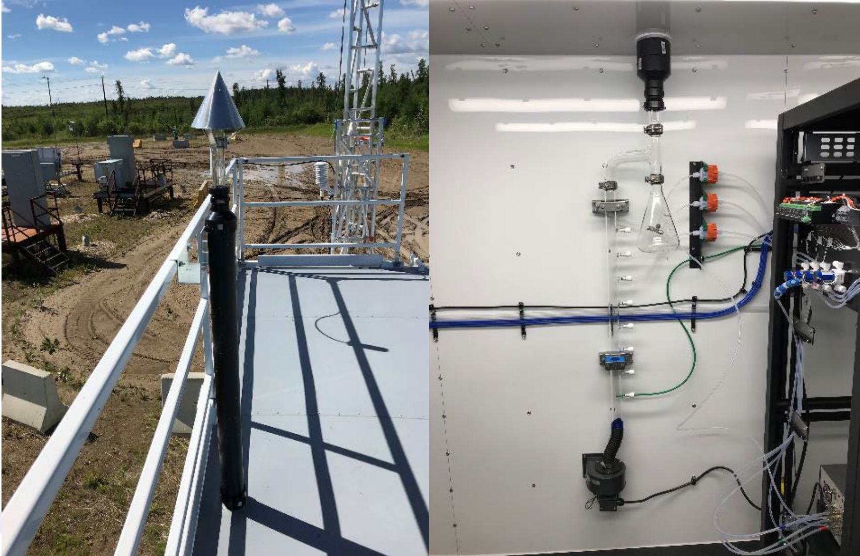
Figure 10 – Photo showing the inlet and sample manifold.
