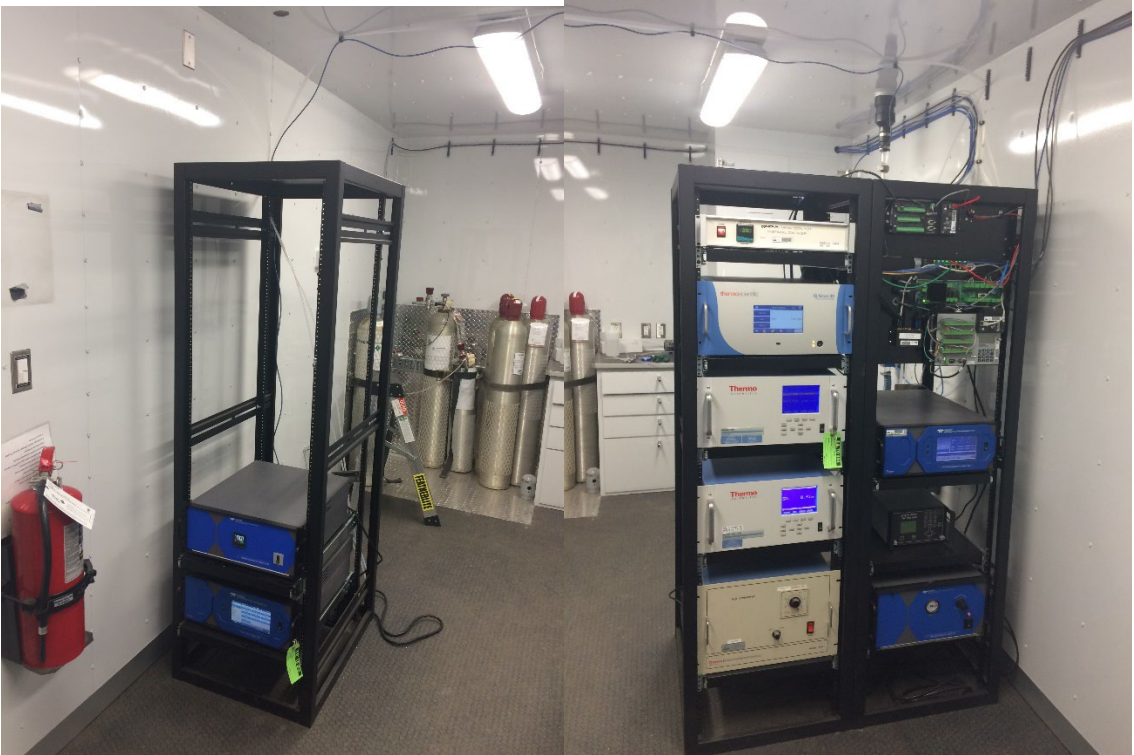
Figure 12 –Photo of the front of instrument rack
