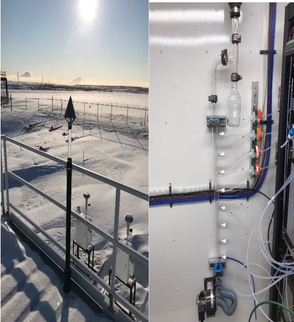
Figure 9 – Photo showing the inlet and sample manifold
