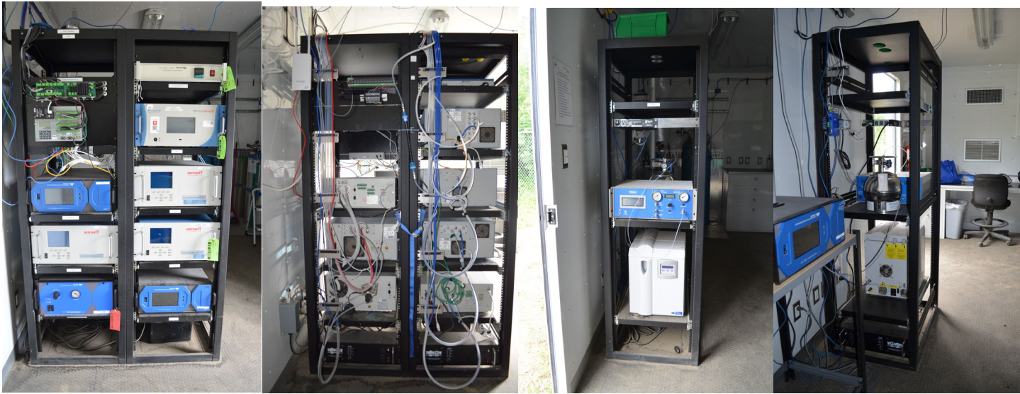
Figure 12 –Photo of the front and the back of instrument rack
