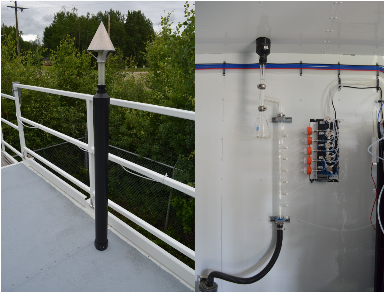
Figure 10 – Photo showing the inlet and sample manifold
