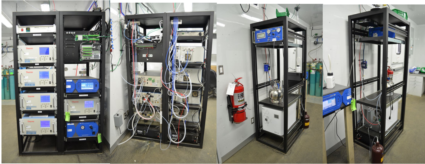
Figure 12 –Photo of front and back of instrument rack
