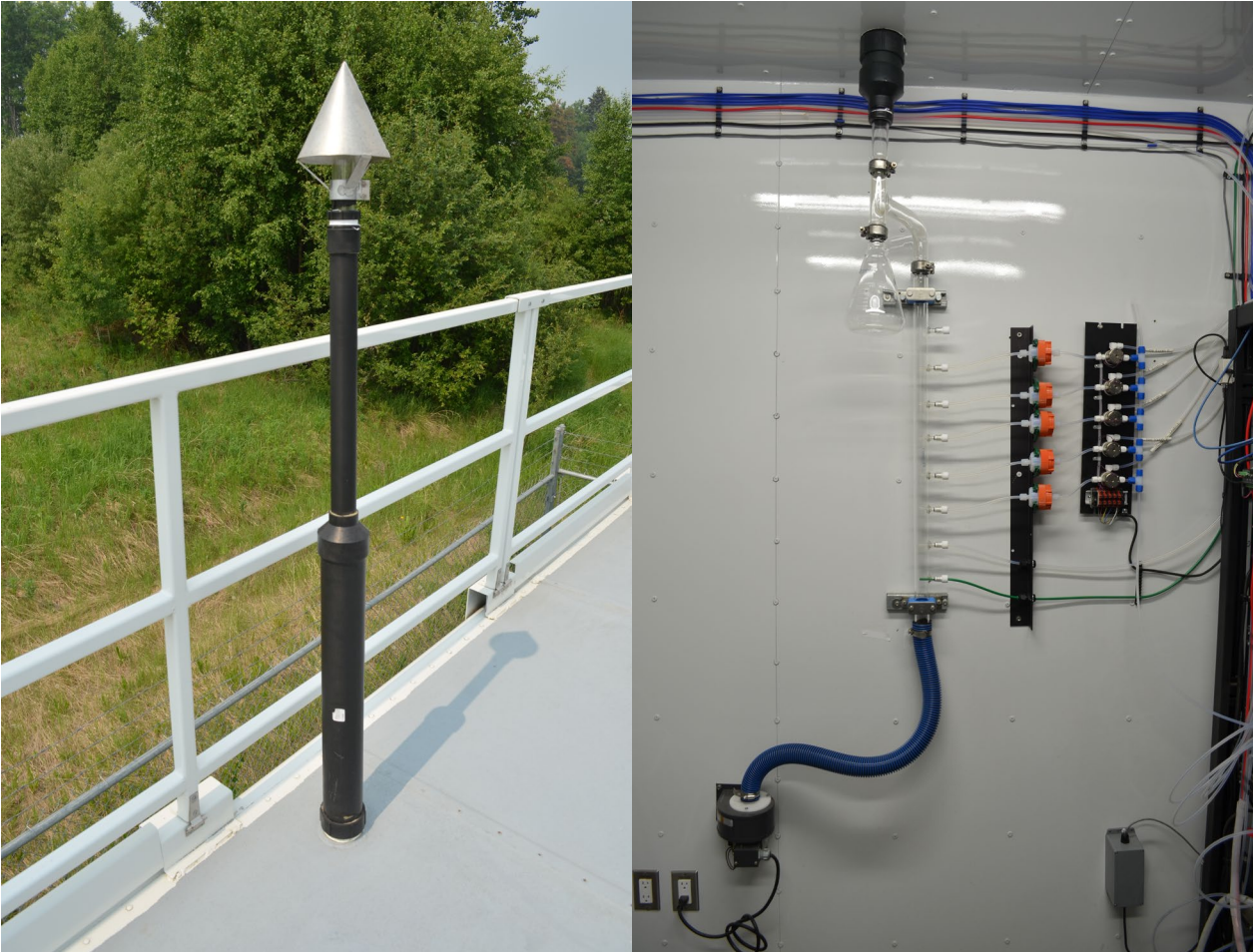
Figure 10 – Photo showing the inlet and sample manifold.
