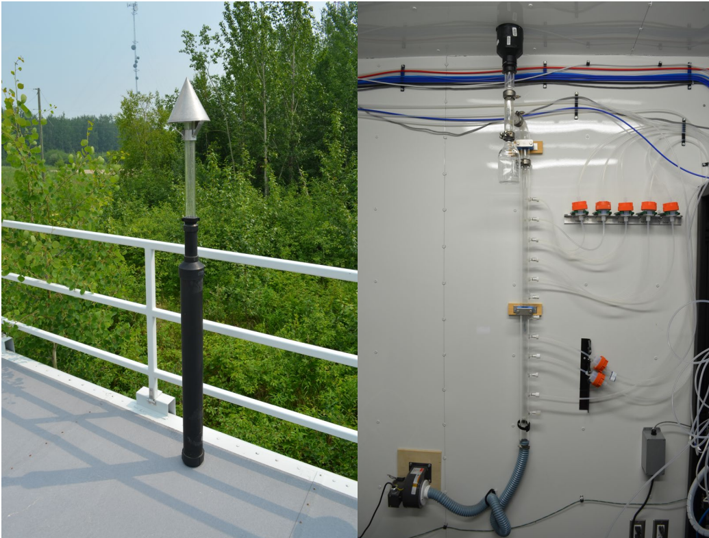
Figure 10 – Photo showing the inlet and sample manifold
