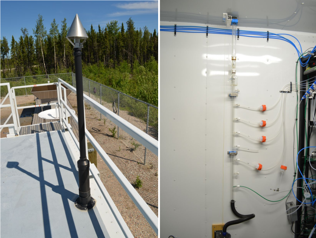
Figure 10 – Photo showing the inlet and sample manifold
