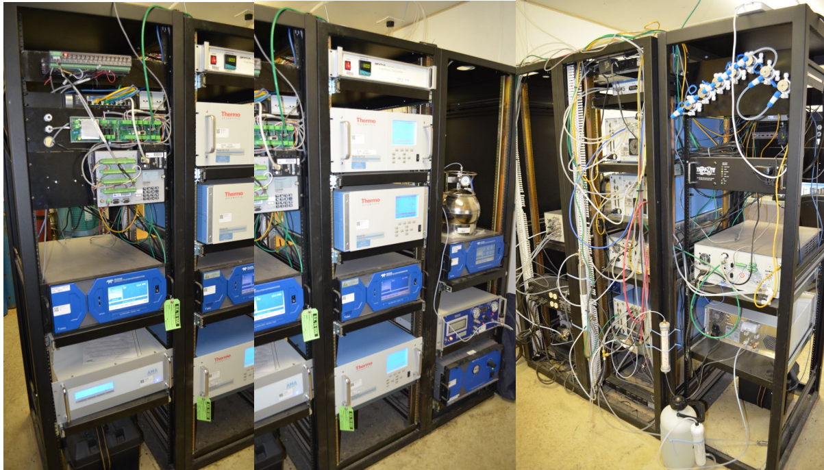
Figure 12 –Photo of the front and the back of instrument rack
