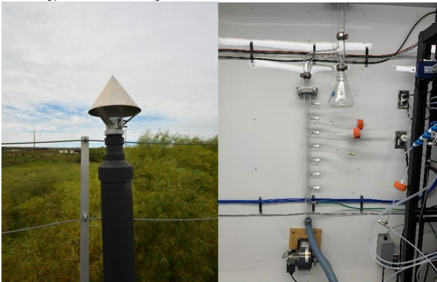
Figure 10 – Photo showing the inlet and sample manifold.
