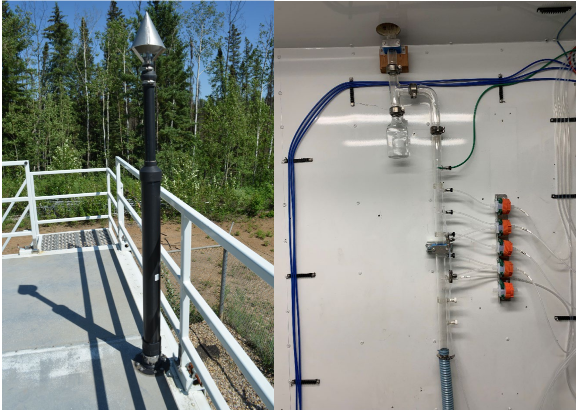
Figure 11 – Photo showing the inlet and sample manifold
