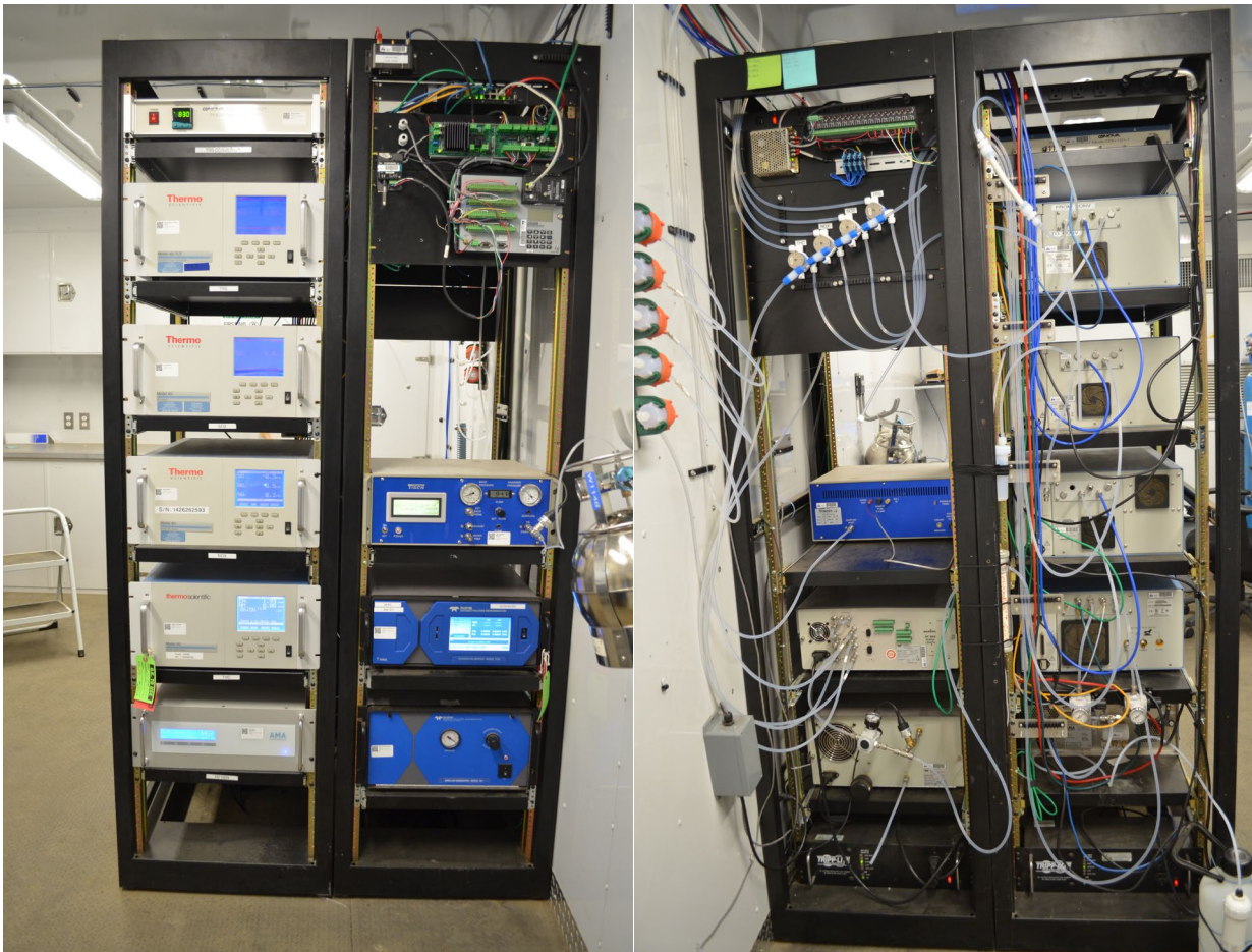
Figure 13 –Photo of the front and the back of instrument rack
