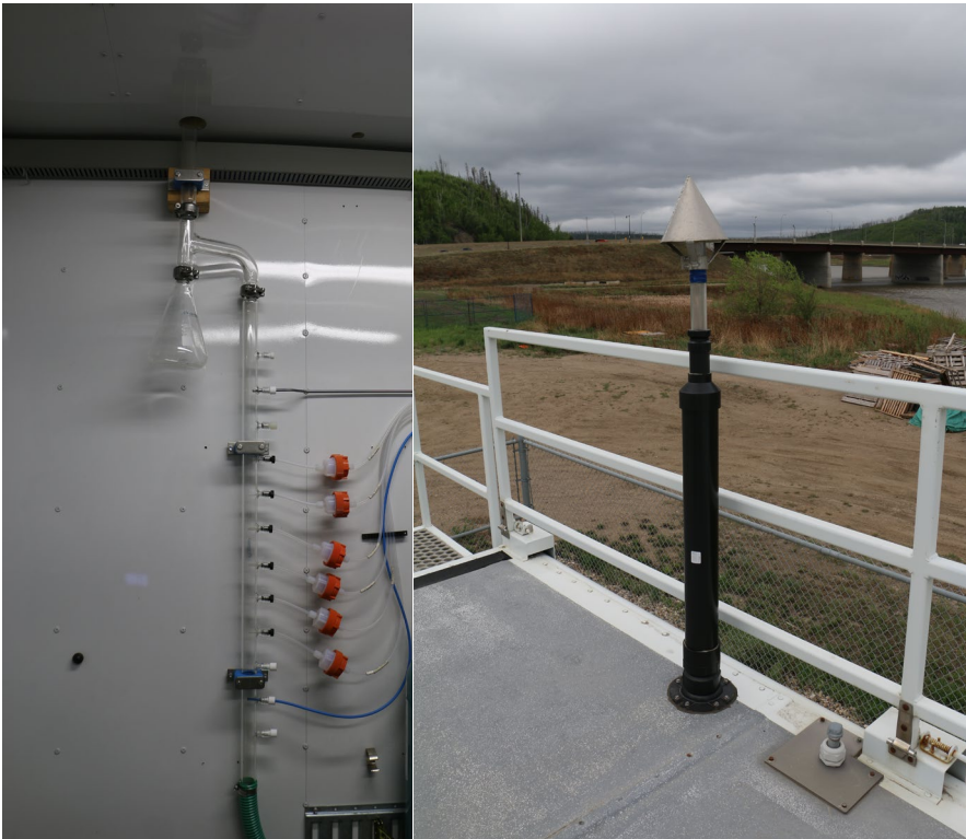
Figure 10 – Photo showing the inlet and sample manifold
