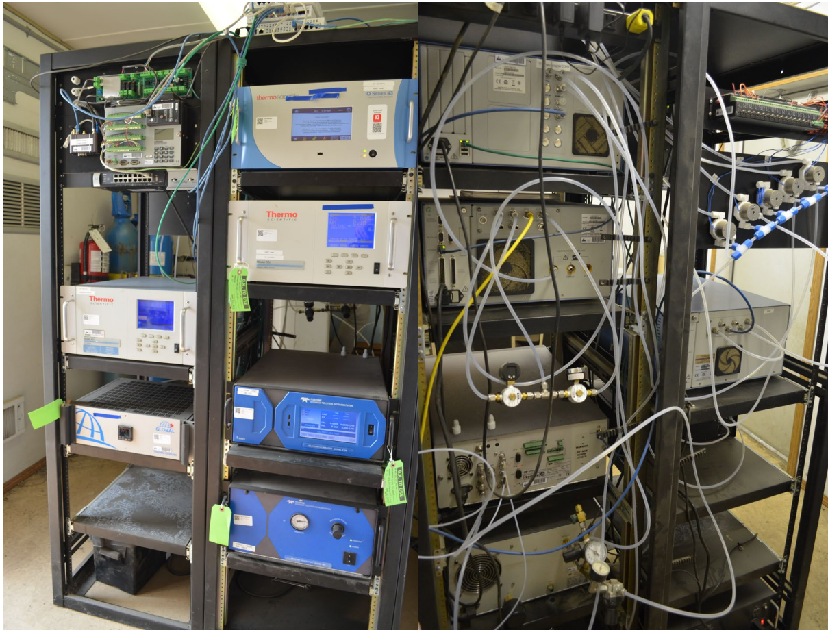
Figure 12 –Photo of the front and the back of instrument rack
