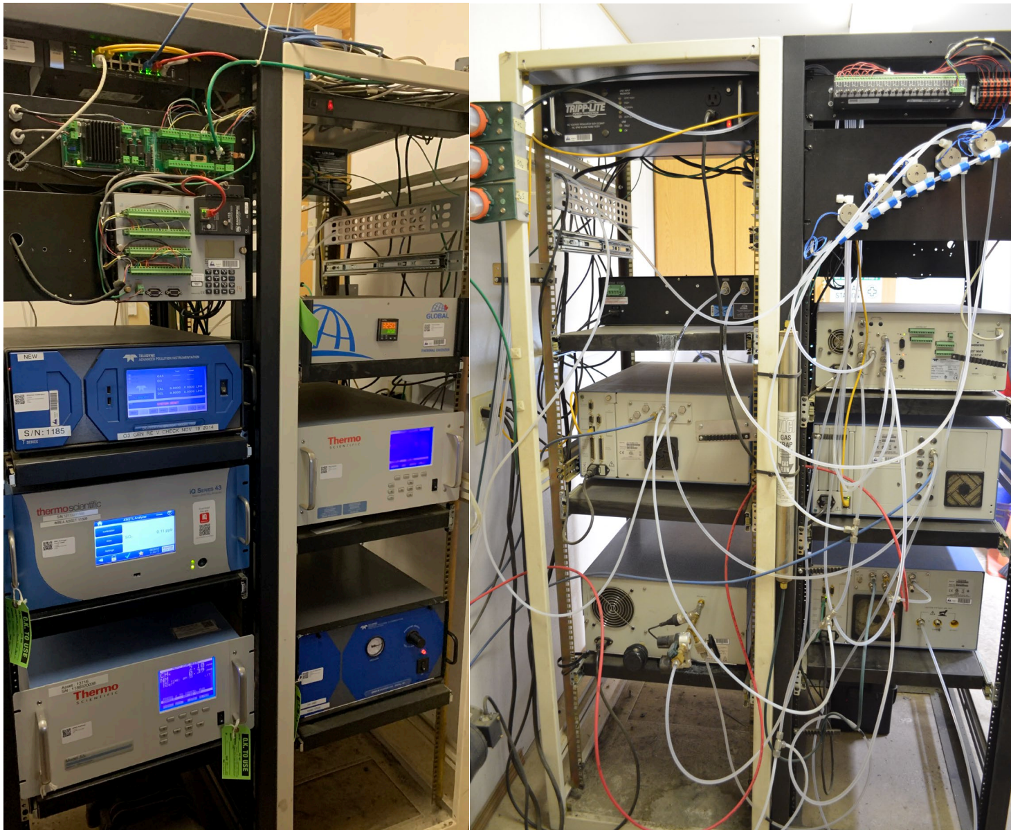
Figure 12 –Photo of the front and the back of instrument rack
