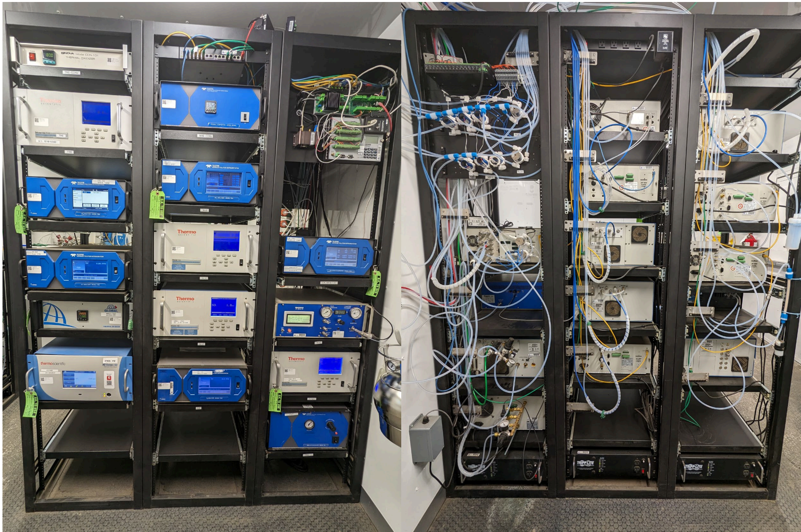
Figure 12 –Photo of the front and the back of the instrument rack
