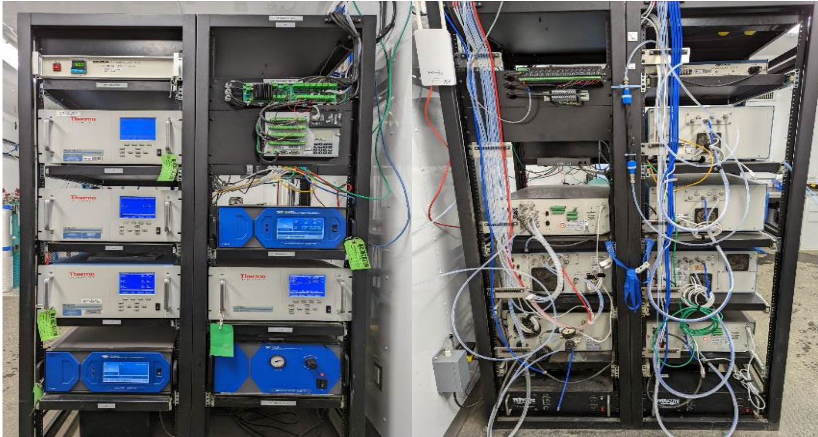
Figure 7.2 –Photo of the front and the back of instrument rack
