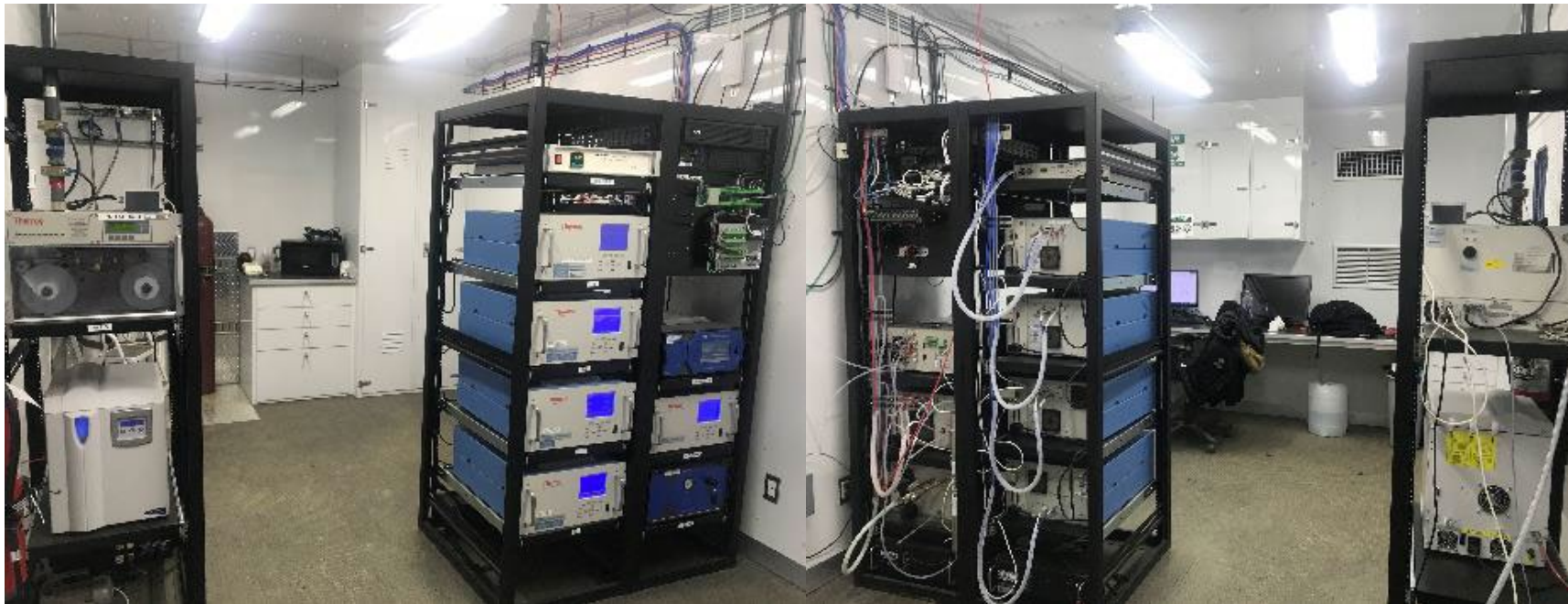
Figure 7.2 –Photo of front and back of instrument rack
