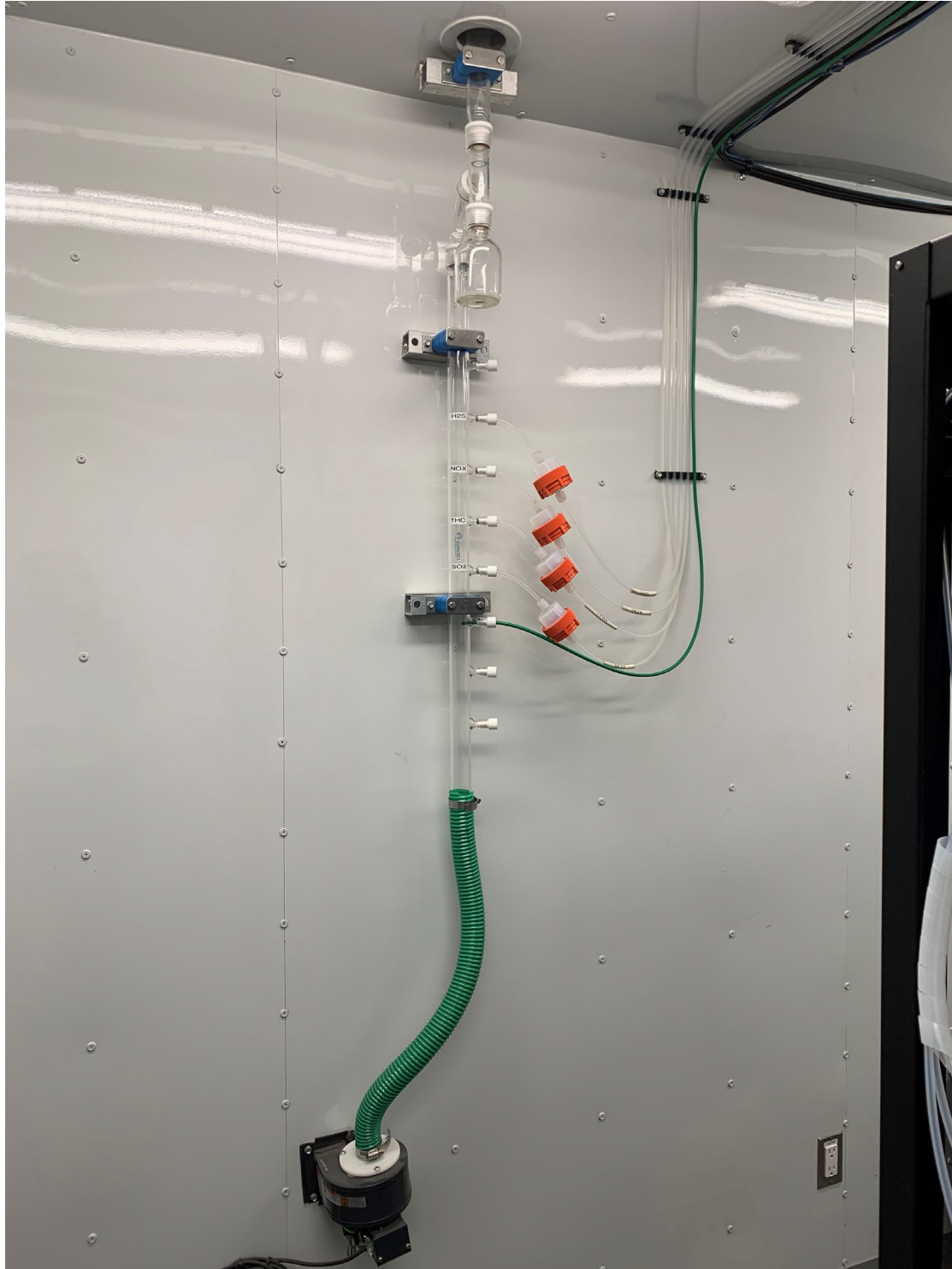
Figure 6.0 – Photo showing the inlet and sample manifold
