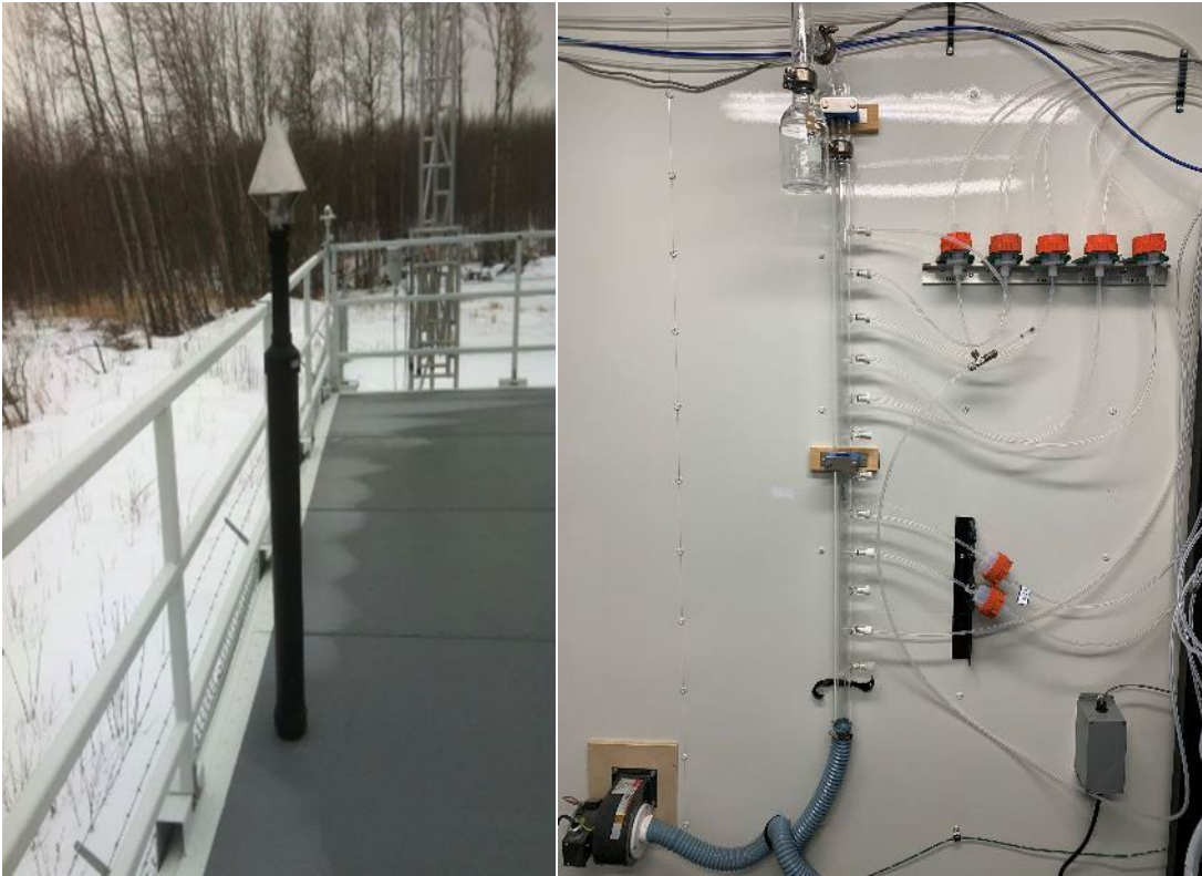
Figure 7.0 – Photo showing the inlet and sample manifold
