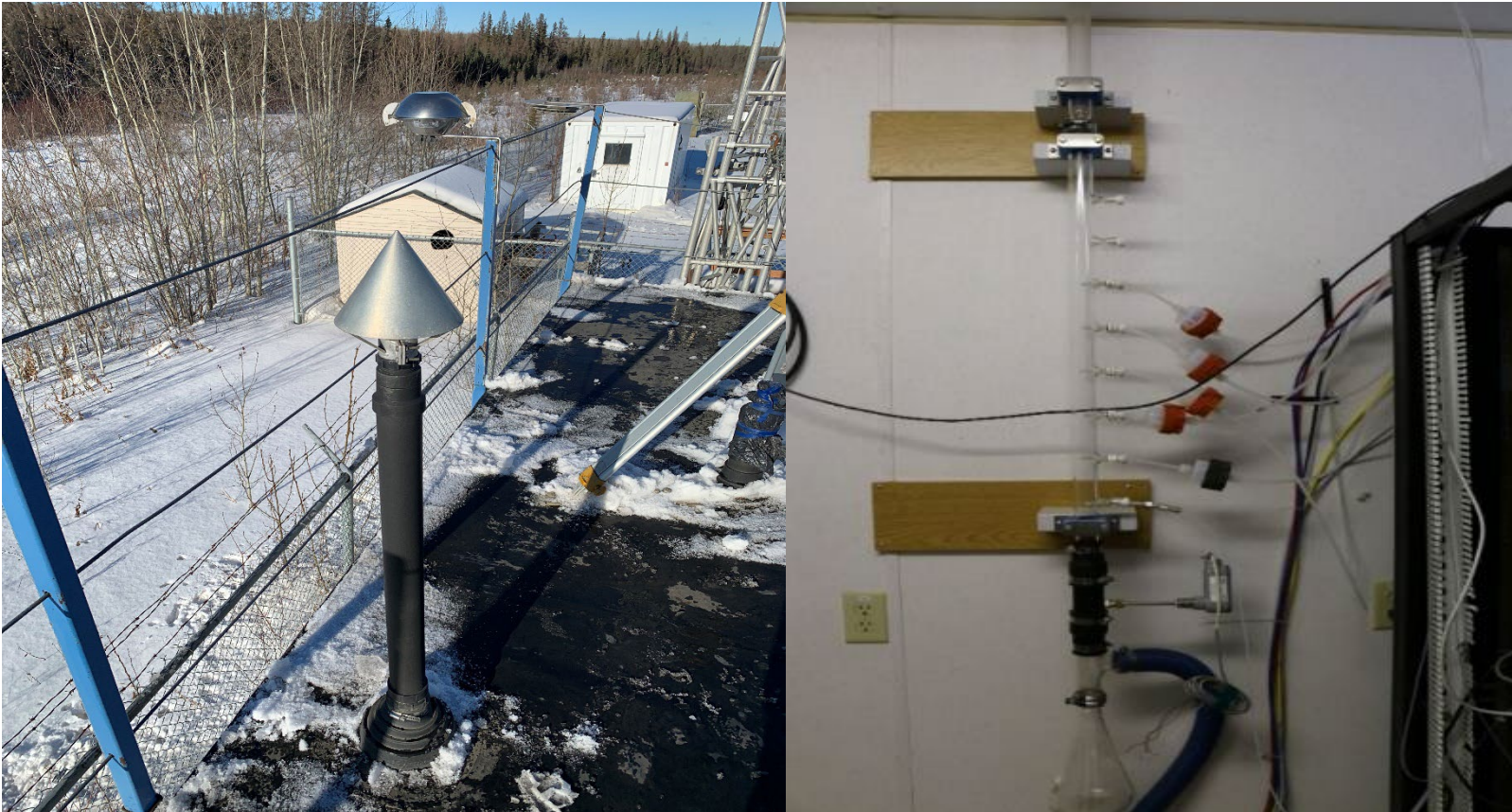
Figure 7.0 – Photo showing the inlet and sample manifold.
