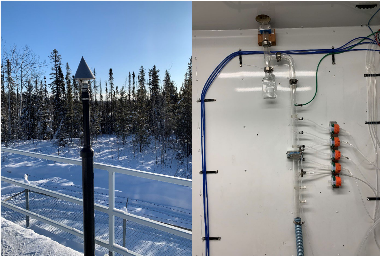
Figure 7.0 – Photo showing the inlet and sample manifold
