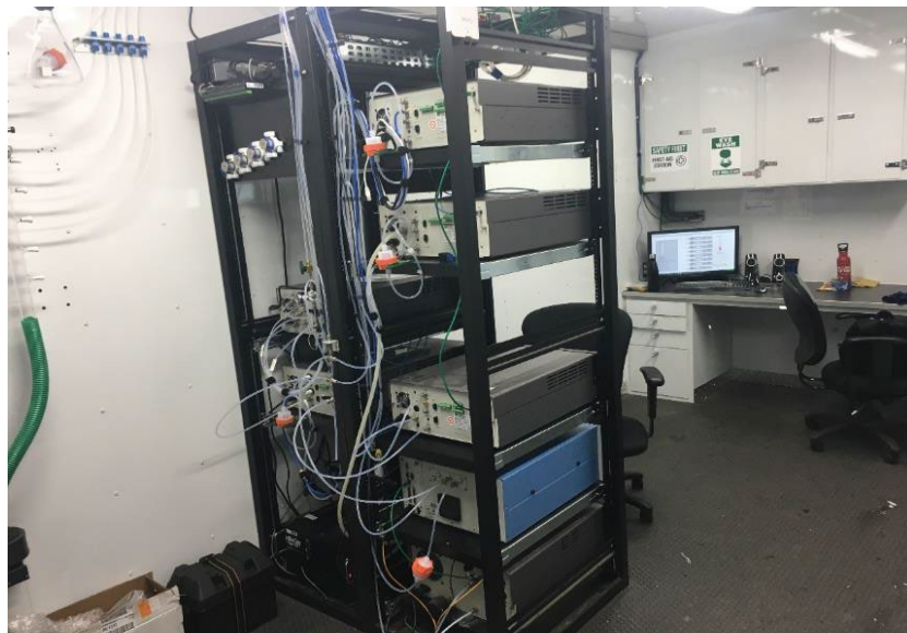
Figure 6.2 –Photo of the front and the back of instrument rack
