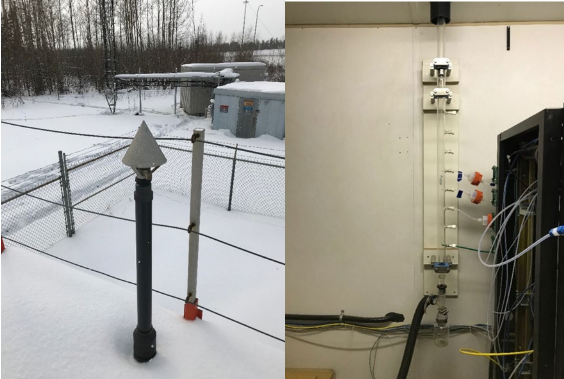
Figure 7.0 – Photo showing the inlet and sample manifold
