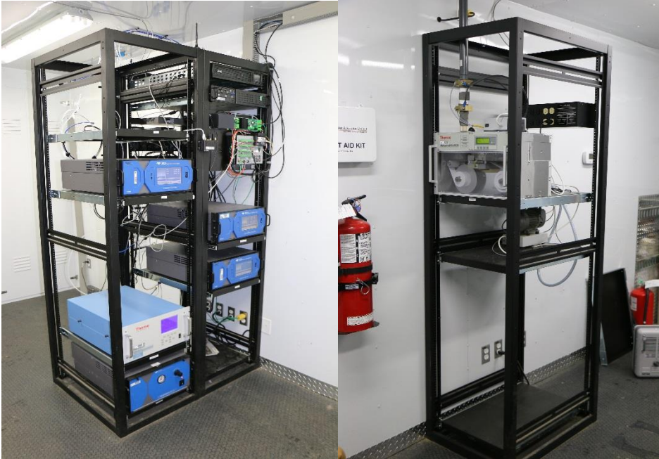
Figure 4.6 – East Rack (on the left) & West Rack
