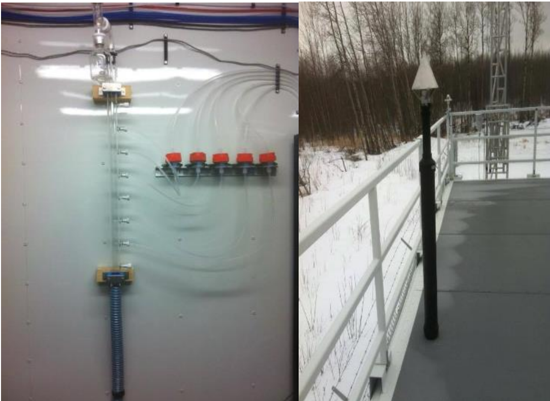
Figure 4.5 – Indoor sample manifold setup and outdoor sample inlet
