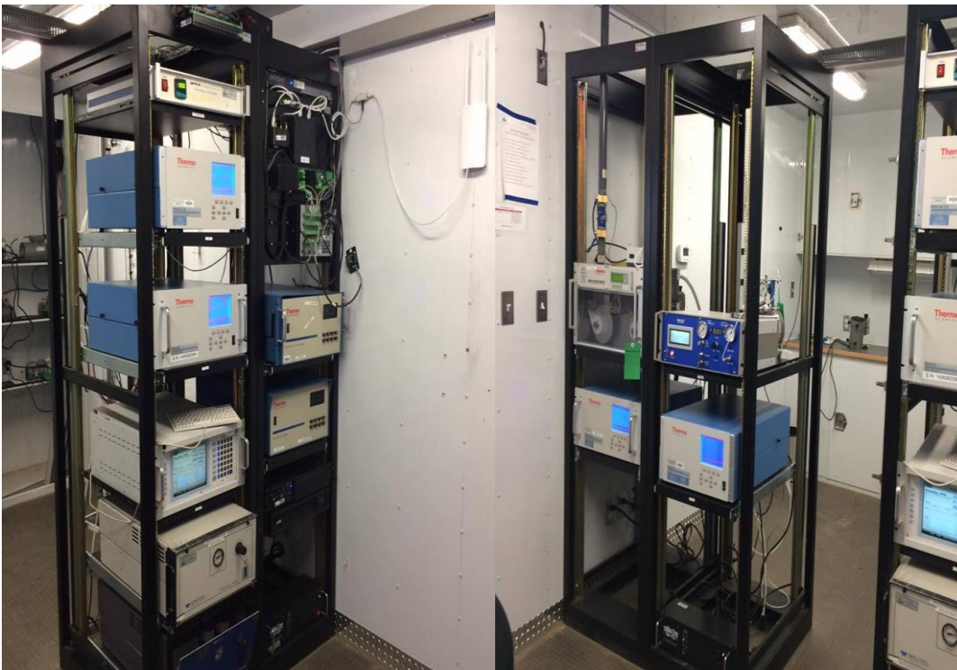
Figure 4.7 – East Rack (on the left) & West Rack
