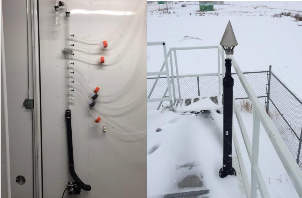
Figure 4.6 –Indoor Sample Manifold and Outdoor sample inlet
