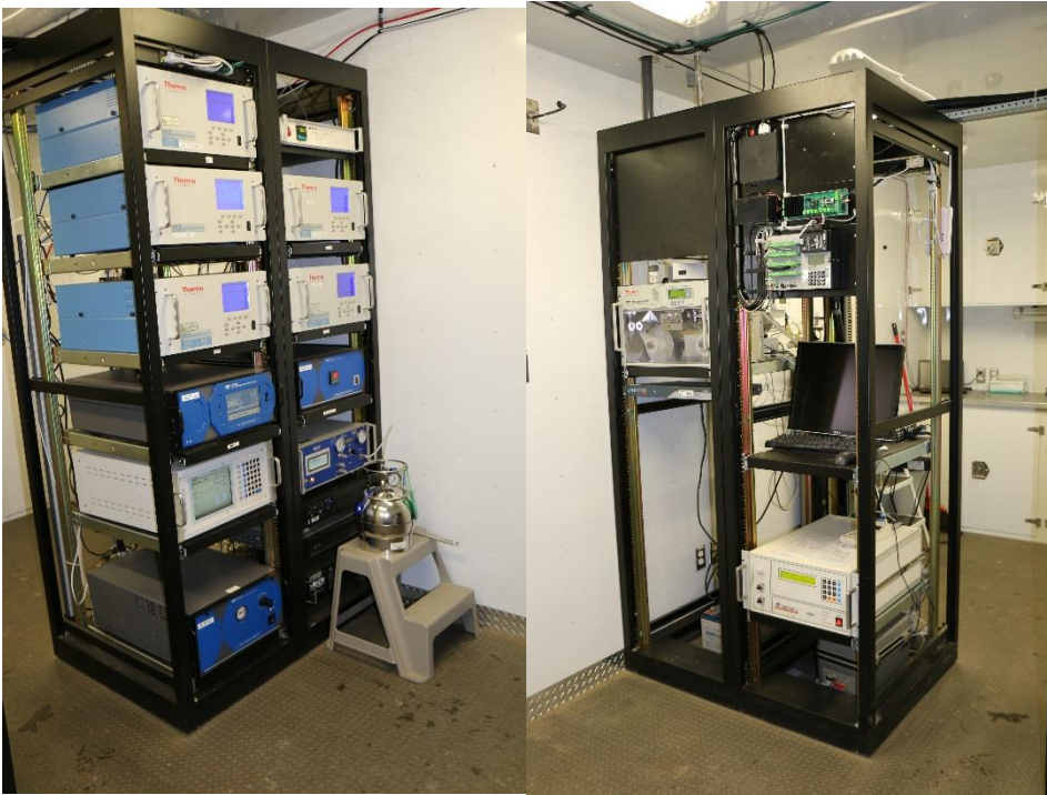
Figure 4.6 – East (on left side) and west instrument racks
