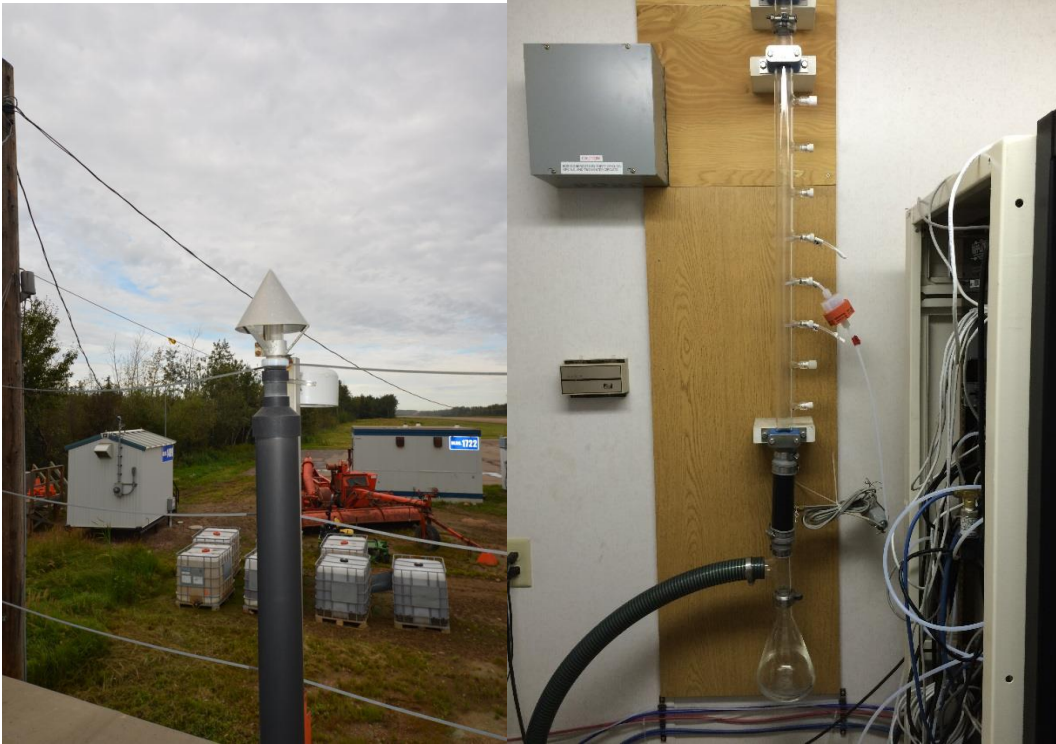
Figure 4.6 – Outdoor Sample Inlet and Indoor manifold setup
