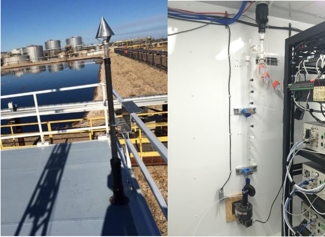
Figure 4.6 – Outdoor Sample Inlet and Indoor manifold setup
