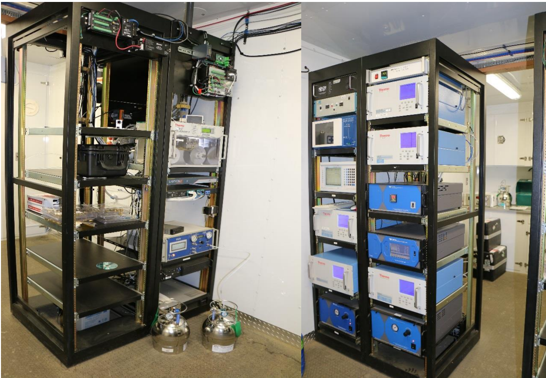
Figure 4.11 – East Rack (on the left) & West Rack
