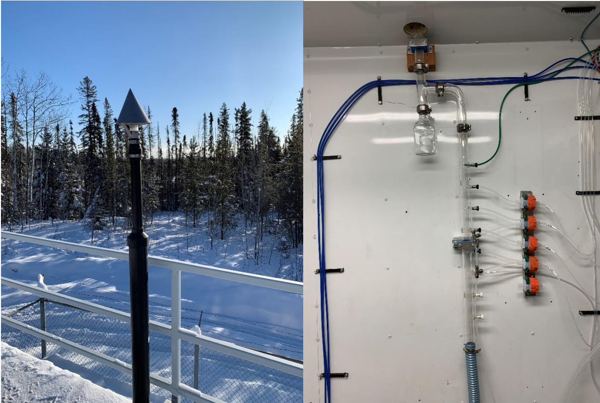
Figure 7.0 – Photo showing the inlet and sample manifold
