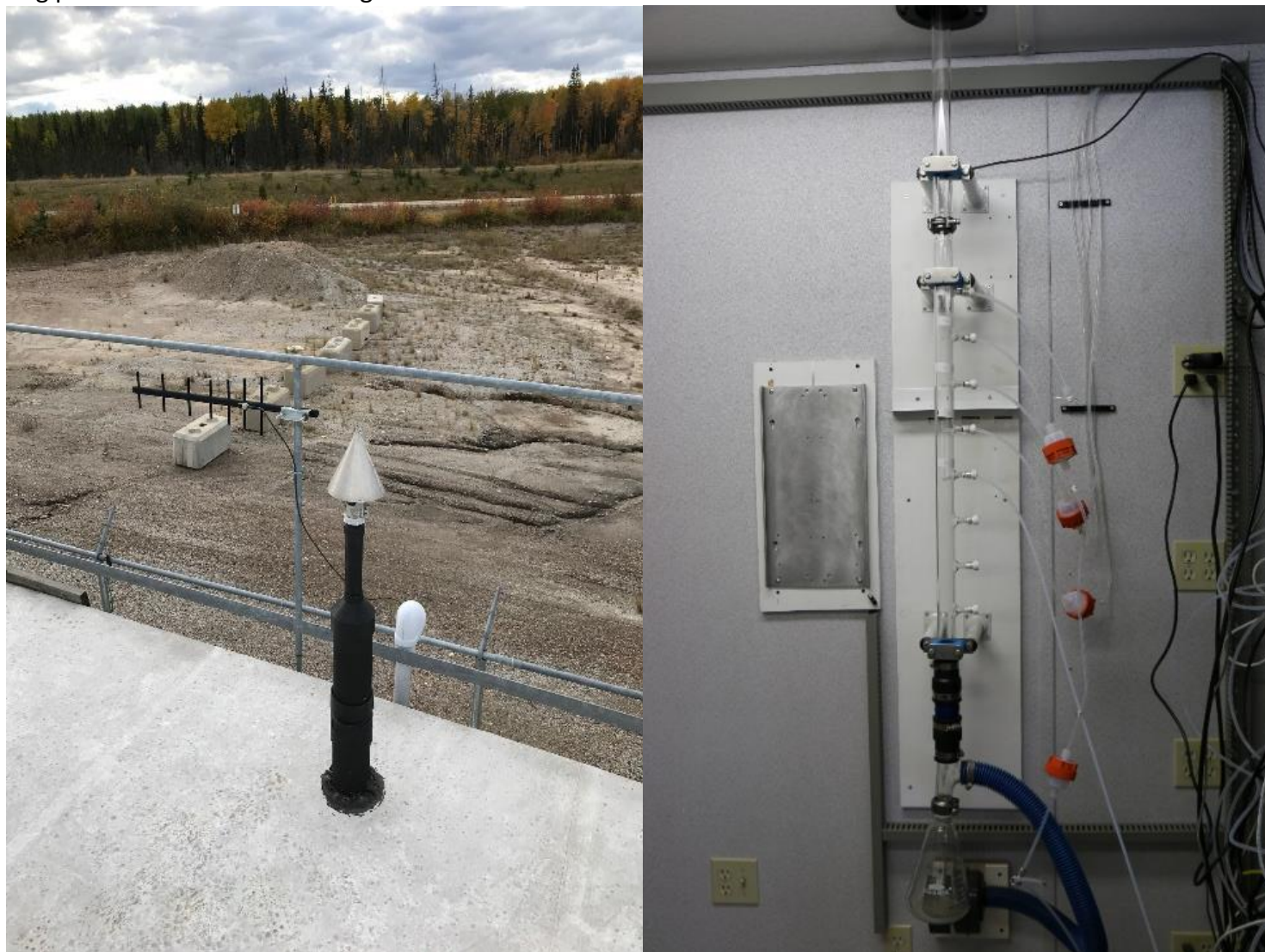
Figure 7.0 – Photo showing the inlet and sample manifold
