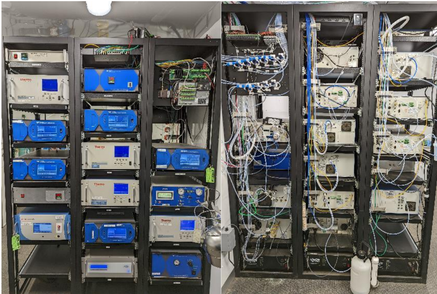
Figure 6.2 –Photo of the front and the back of the right instrument rack
