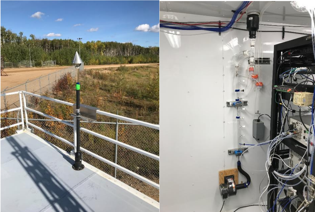
Figure 6.0 – Photo showing the inlet and sample manifold
