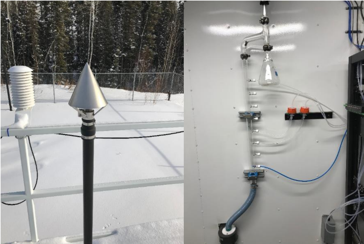
Figure 7.0 – Photo showing the inlet and sample manifold
