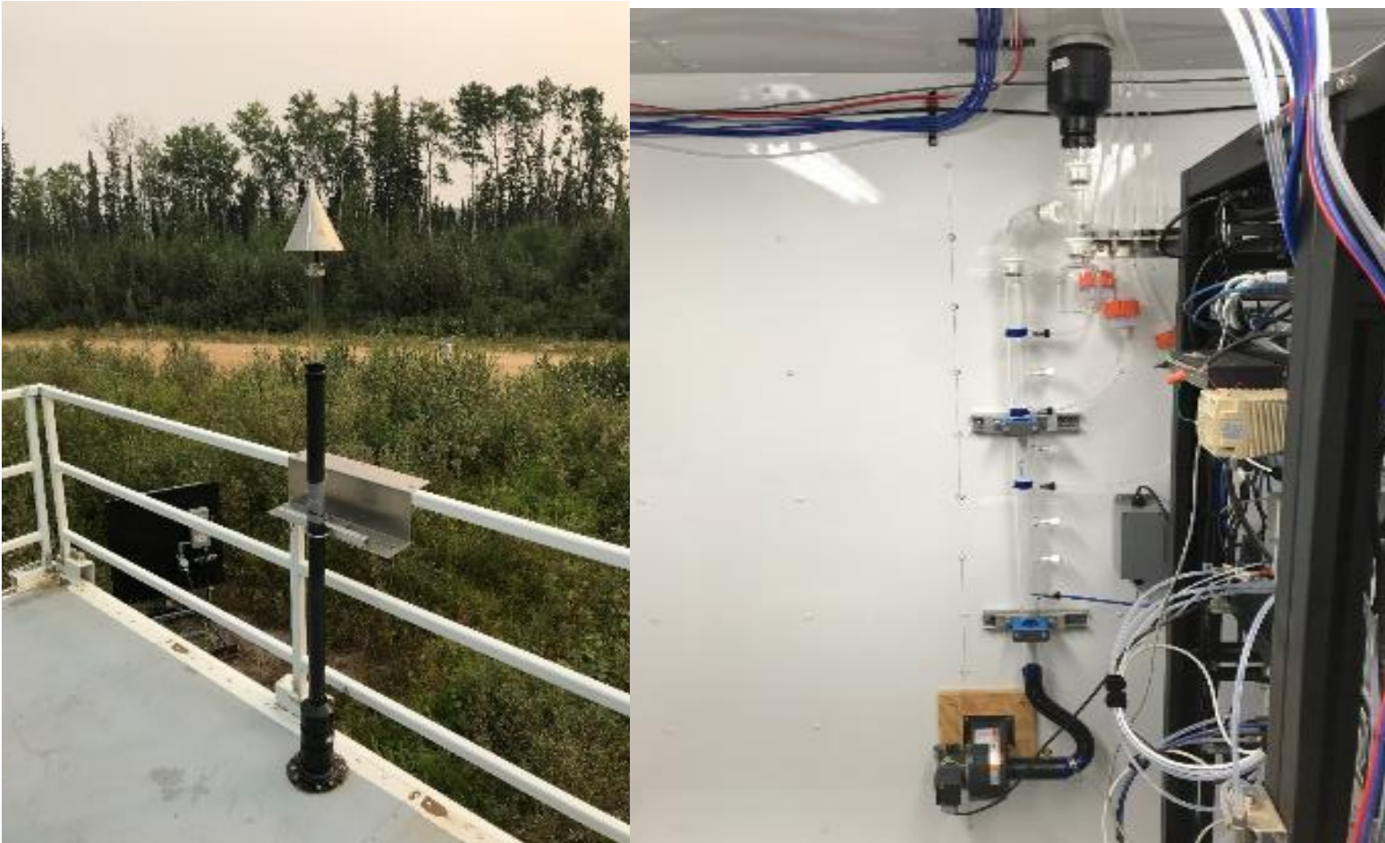
Figure 7.0 – Photo showing the inlet and sample manifold
