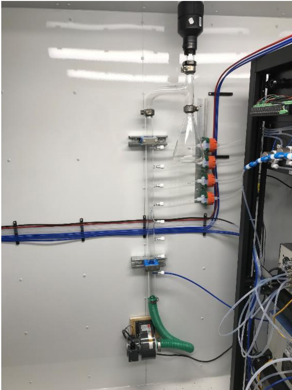
Figure 6.0 – Photo showing the inlet and sample manifold
