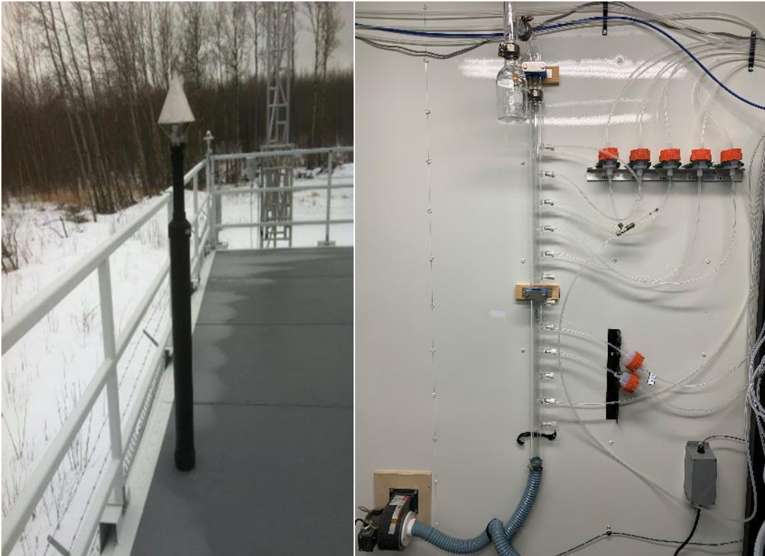
Figure 7.0 – Photo showing the inlet and sample manifold
