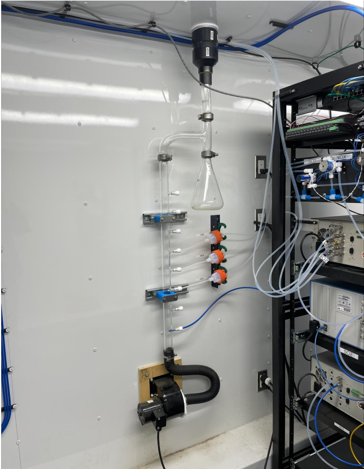
Figure 7.0 – Photo showing the inlet and sample manifold.
