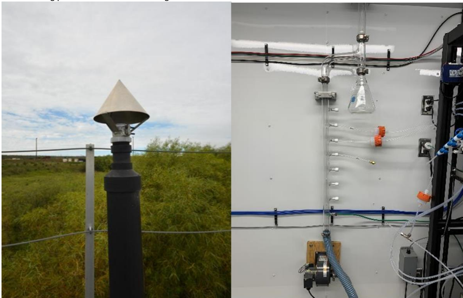
Figure 7.0 – Photo showing the inlet and sample manifold
