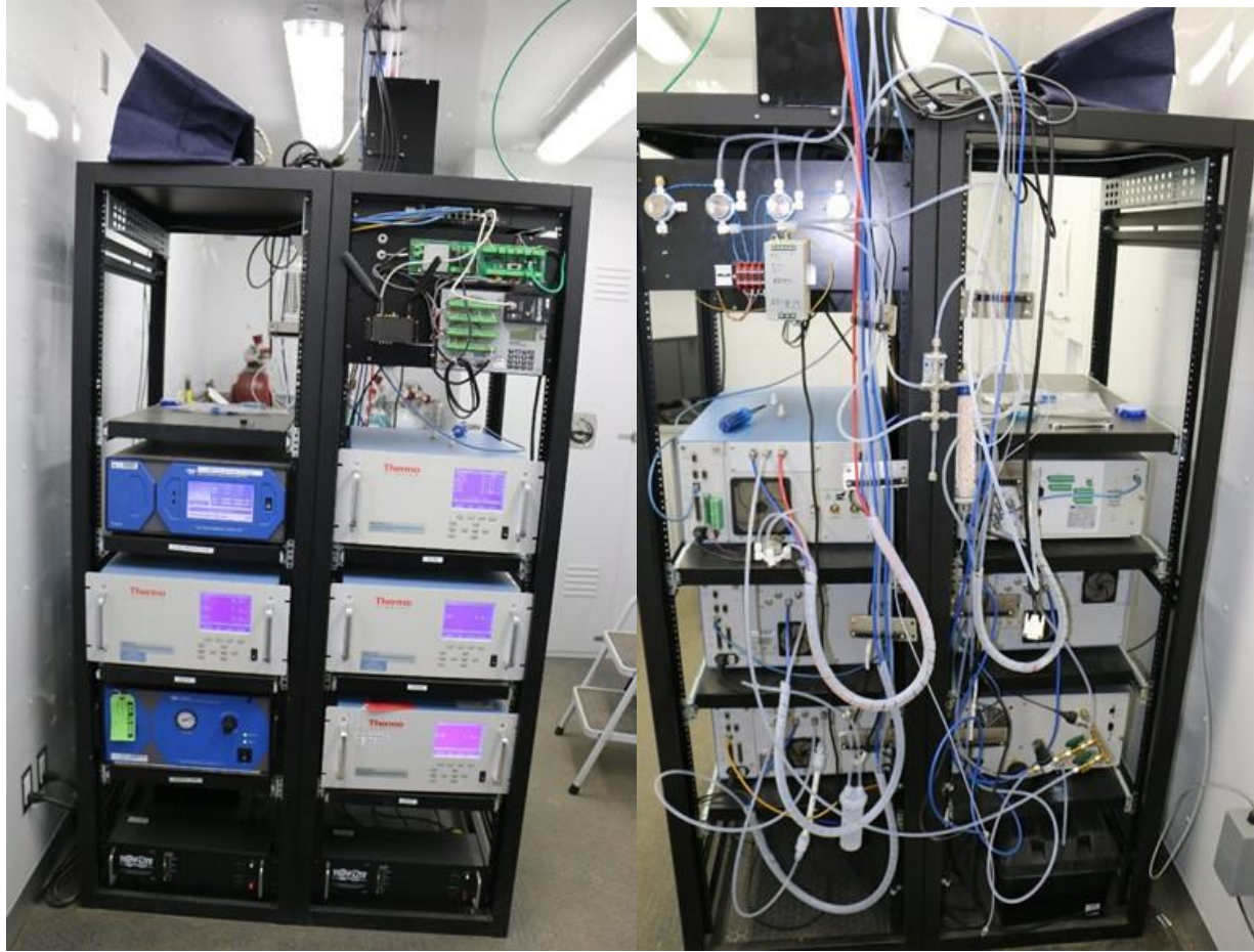
Figure 6.2 –Photo of front and back of instrument rack
