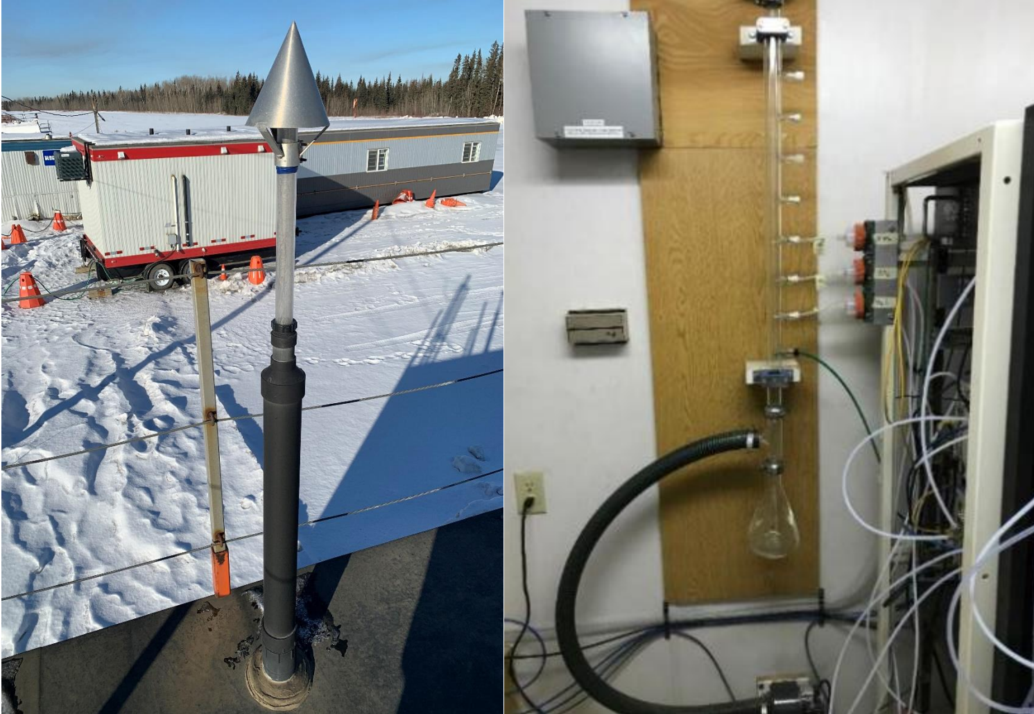
Figure 7.0 – Photo showing the inlet and sample manifold
