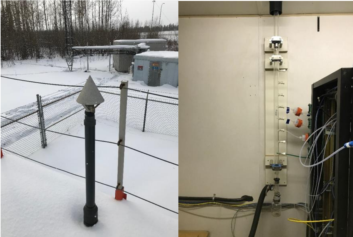
Figure 7.0 – Photo showing the inlet and sample manifold
