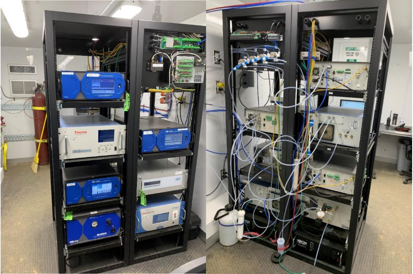
Figure 6.2 –Photo of the front and the back of instrument rack
