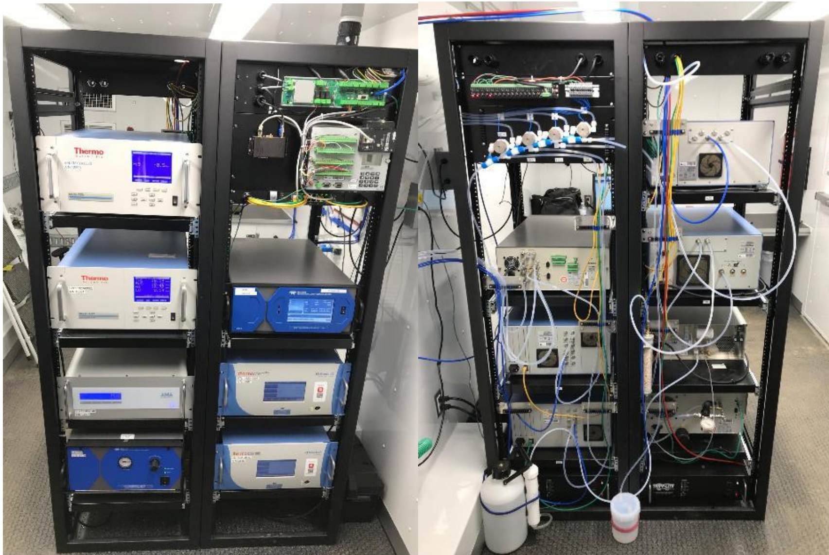
Figure 6.2 –Photo of front and back of instrument rack
