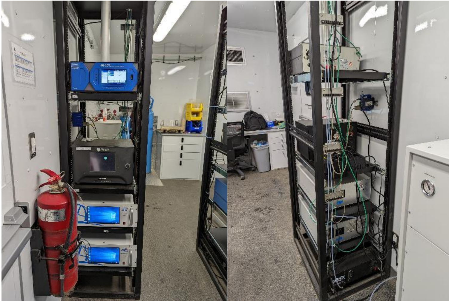
Figure 6.3 –Photo of the front and the back of the left instrument rack
