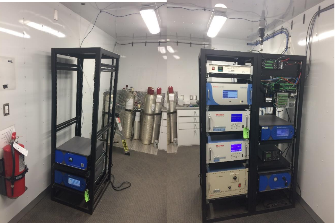
Figure 7.2 –Photo of the front of instrument rack
