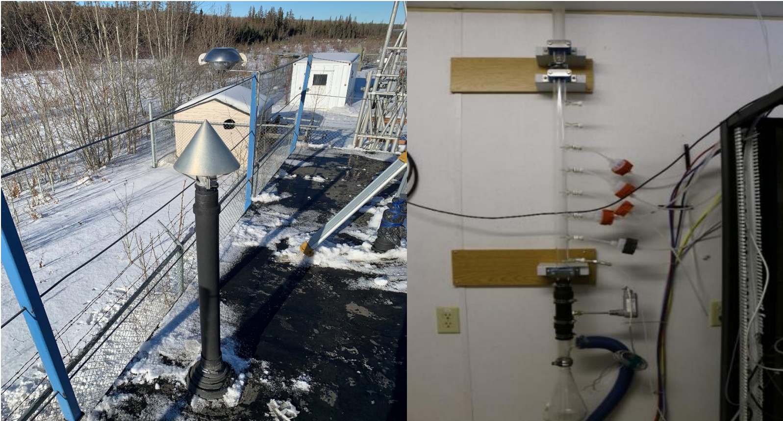
Figure 7.0 – Photo showing the inlet and sample manifold.
