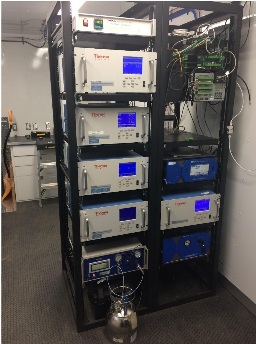
Figure 7.2 –Photo of the front and the back of instrument rack
