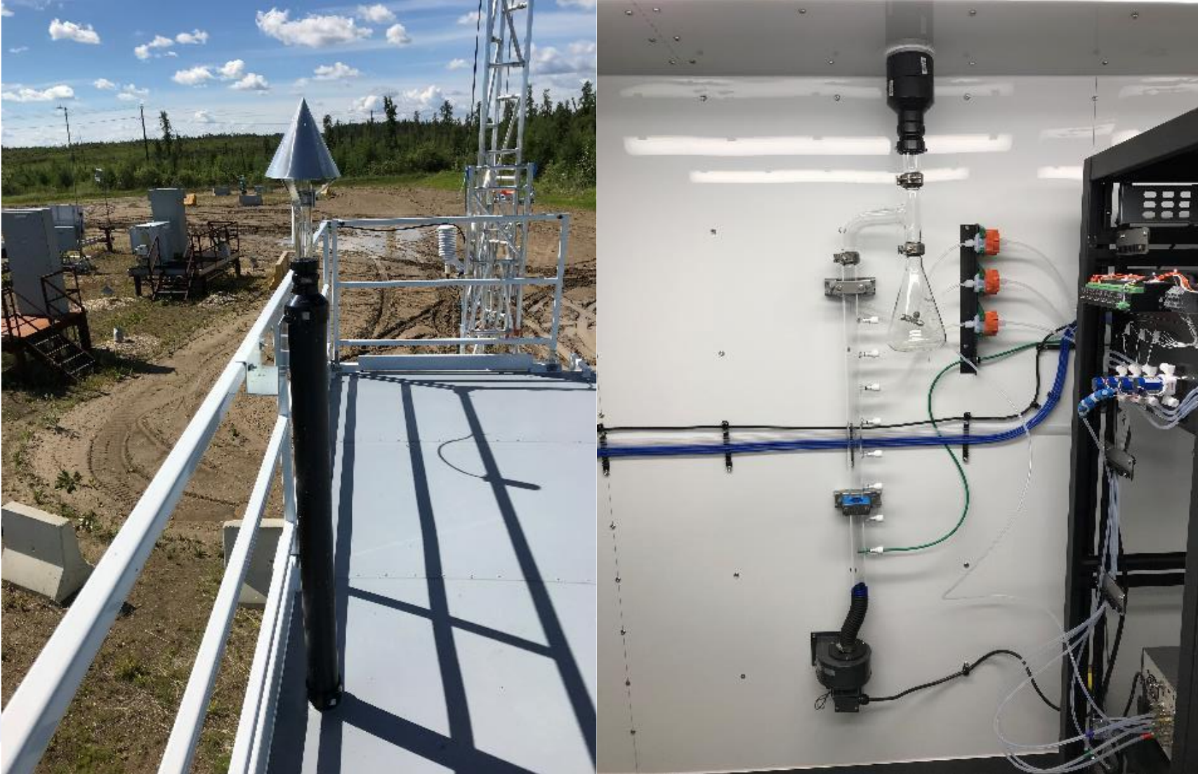
Figure 7.0 – Photo showing the inlet and sample manifold.
