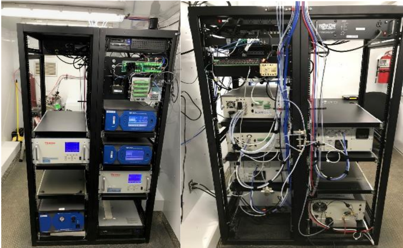
Figure 7.2 –Photo of the front and the back of instrument rack
