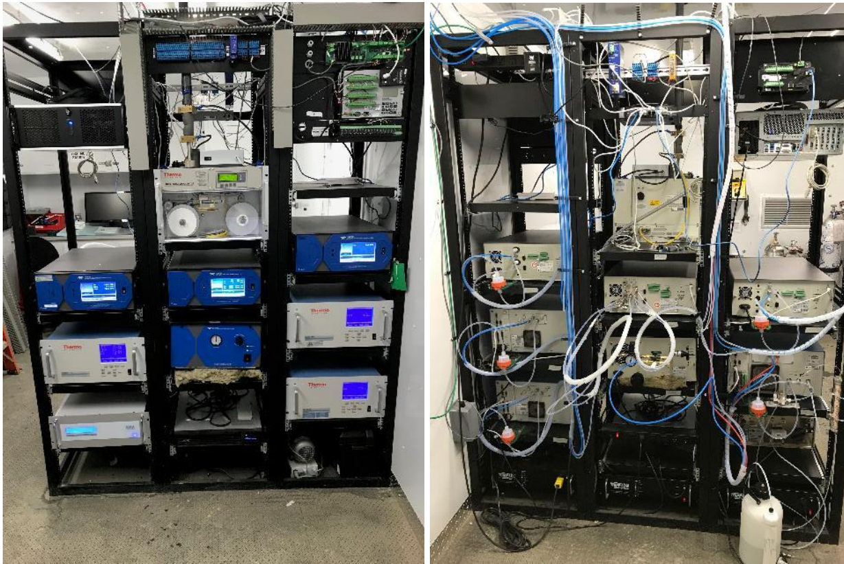
Figure 7.2 –Photo of the front and the back of instrument rack
