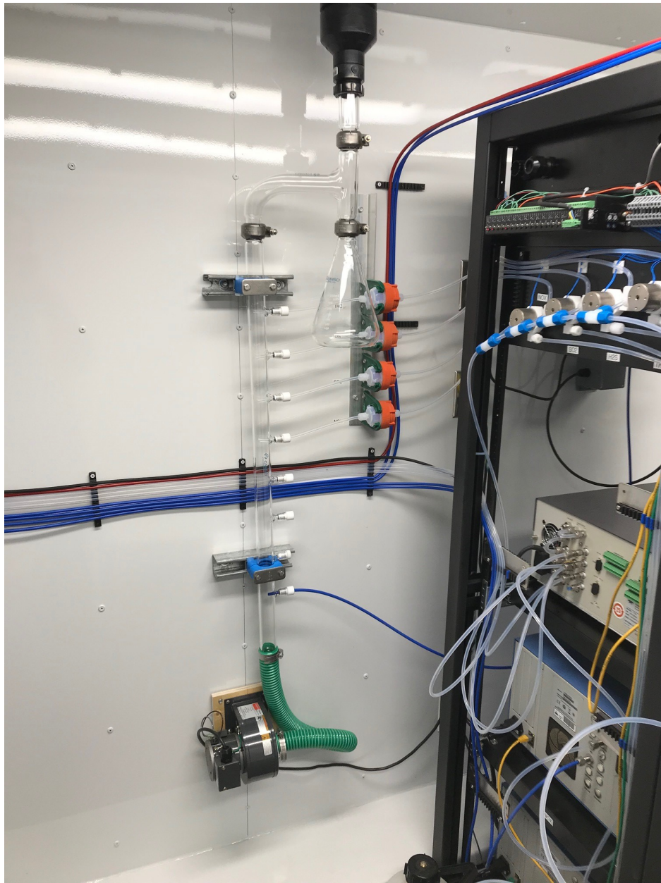
Figure 6.0 – Photo showing the inlet and sample manifold
