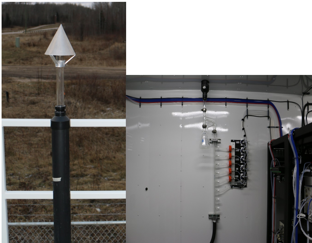
Figure 6.0 – Photo showing the inlet and sample manifold
