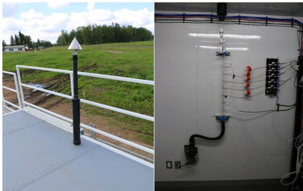
Figure 6.0 – Photo showing the inlet and sample manifold
