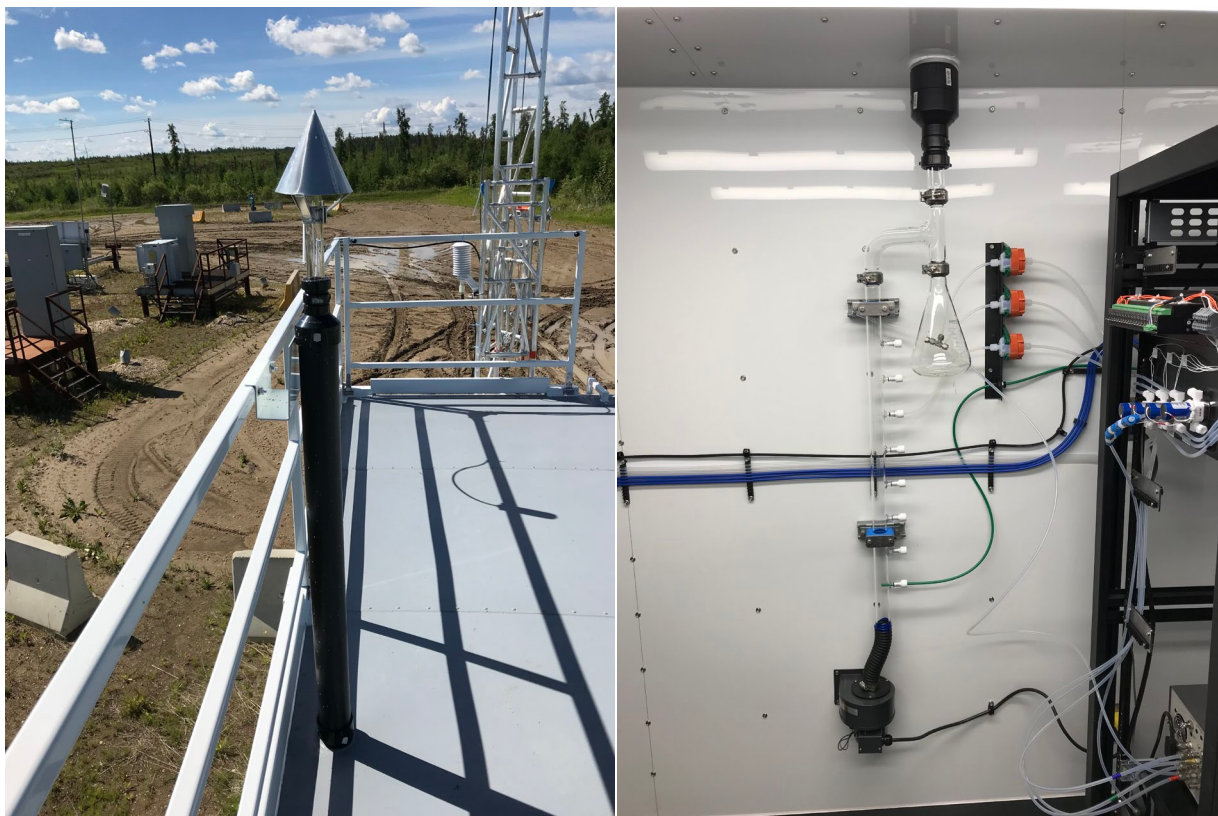
Figure 6.0 – Photo showing the inlet and sample manifold
