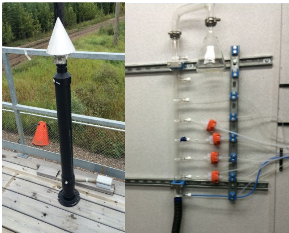
Figure 6.0 – Photo showing the inlet and sample manifold
