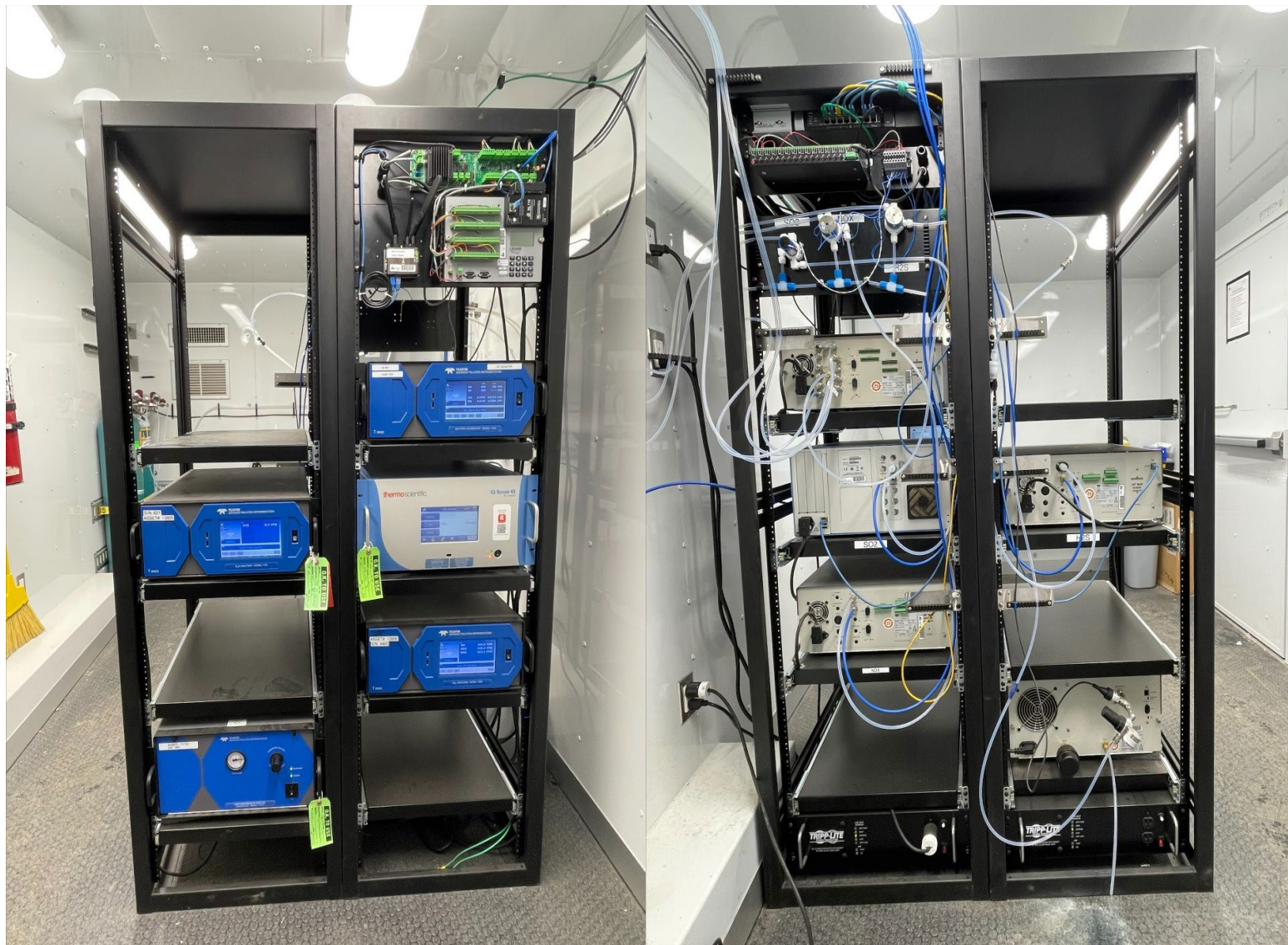
Figure 7.2 –Photo of the front and the back of instrument rack
