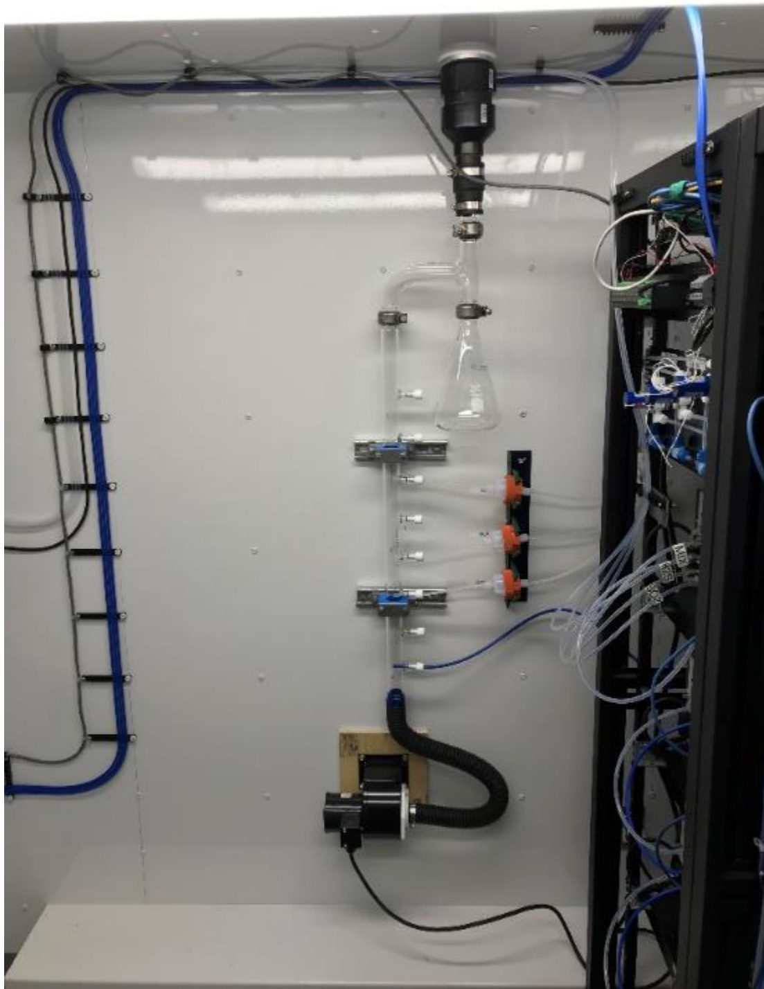
Figure 6.0 – Photo showing the inlet and sample manifold
